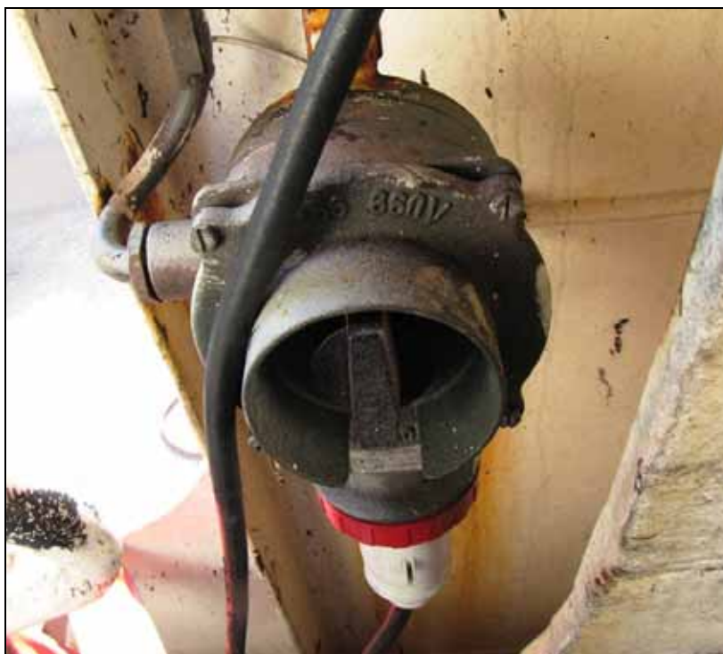
Figure 39: Slightly thermally stressed socket with an inserted plug (deck 6, lane 8)
