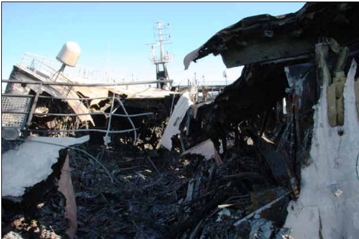
Figure 16: Destroyed accommodation decks, view from deck 7 to the bow
