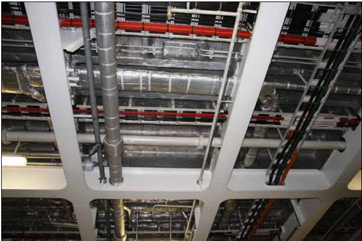
Figure 61: A-60 insulation on deck 6 of the sister vessel, DANA SIRENA
