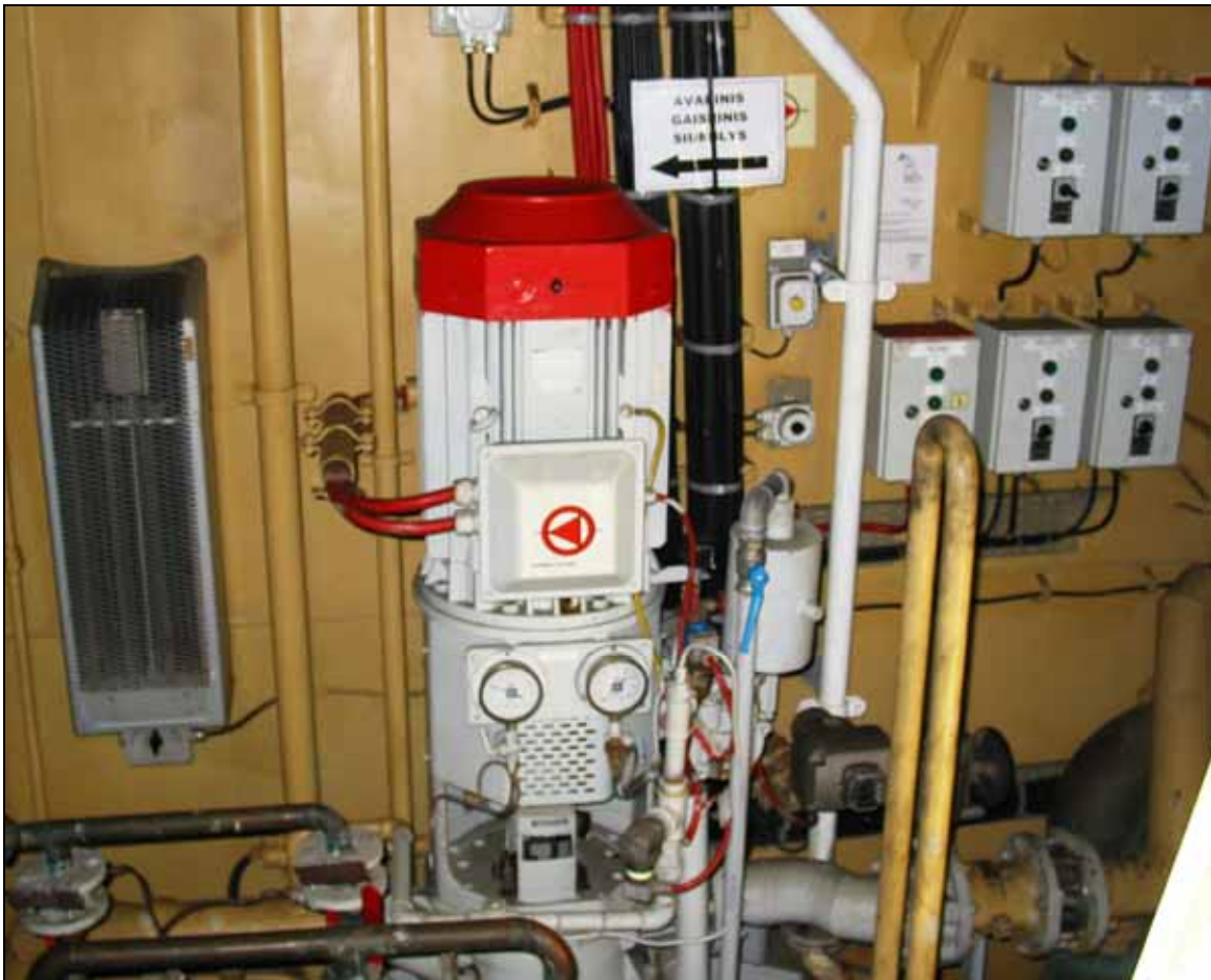
Figure 90: Emergency fire pump in the forward section of the LISCO GLORIA
