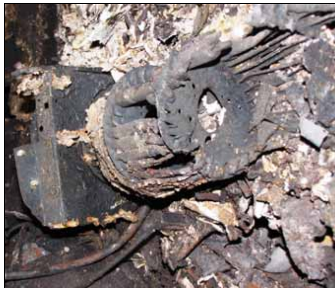
Figure 37: Remains of the refrigeration unit fan
