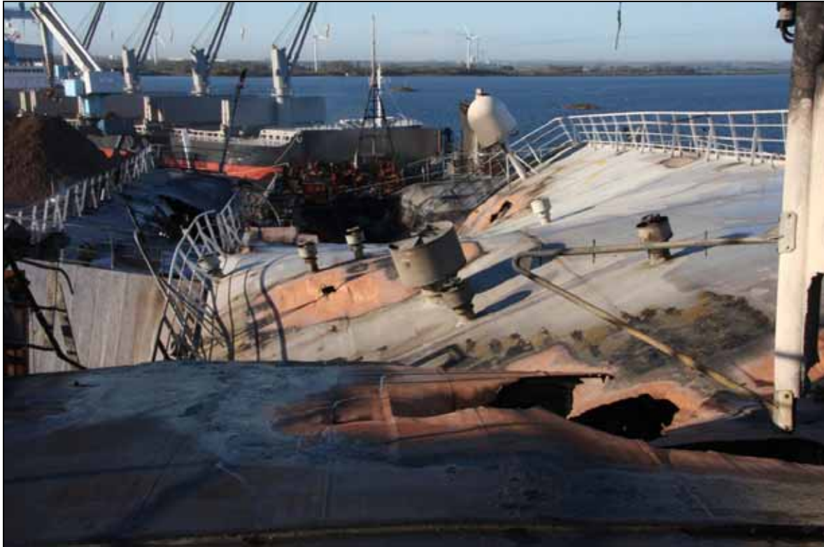
Figure 15: Structural damage in the superstructure, view from observation deck to the stern
