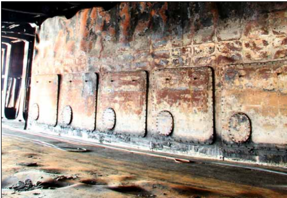
Figure 74: Entrances to the ventilation ducts on deck 6 – port side
