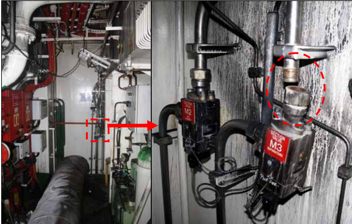
Figure 88: Parted sprinkler system pressure pipe near the engine control room
