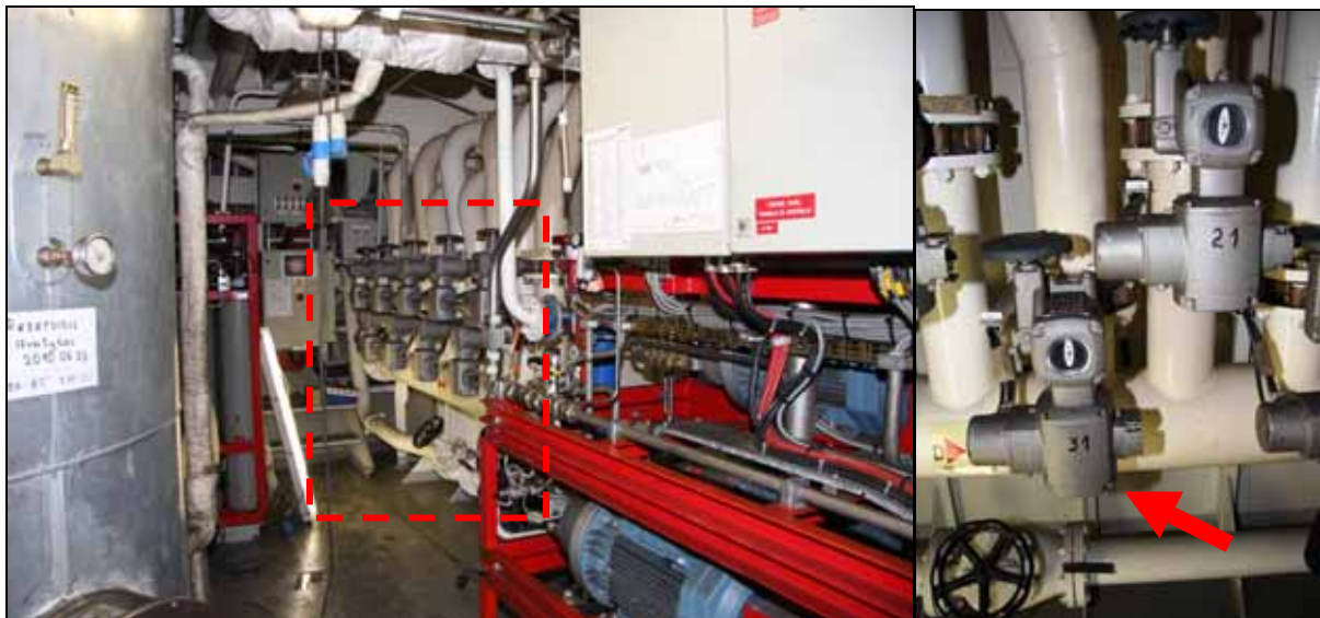
Figure 85: Sprinkler room on board the LISCO GLORIA
