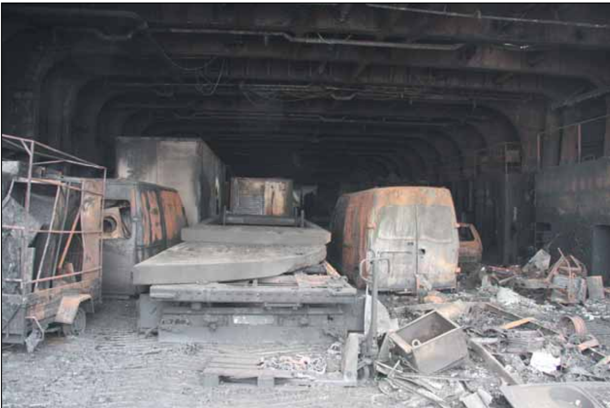
Figure 10: Deck 4 after the fire, looking forward from the stern ramp
