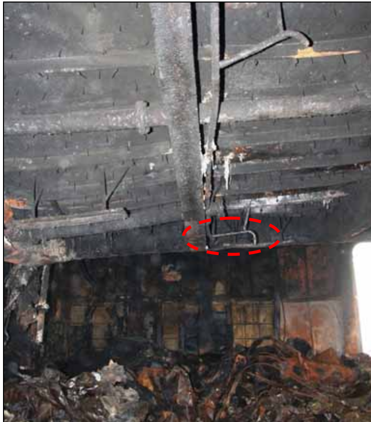
Figure 80: Extinguishing nozzles on the upper deck after the fire
