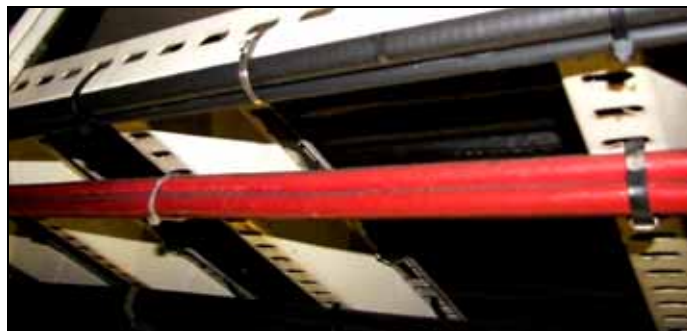
Figure 120: Metal and plastic cable ties used on board the DANA SIRENA
