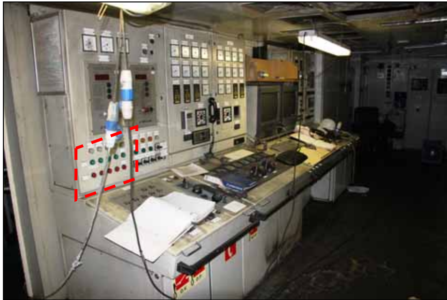
Figure 81: Control panel for the fire and drencher pumps in the engine control room of the LISCO GLORIA
