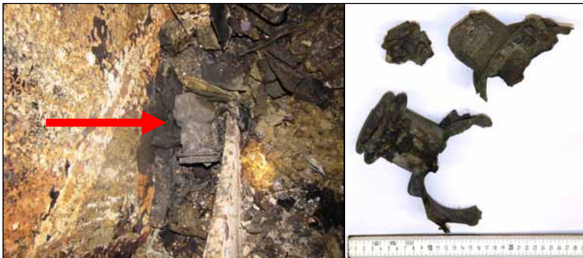
Figure 40: Remains of three-phase current power outlets at frame 200 (starboard)
