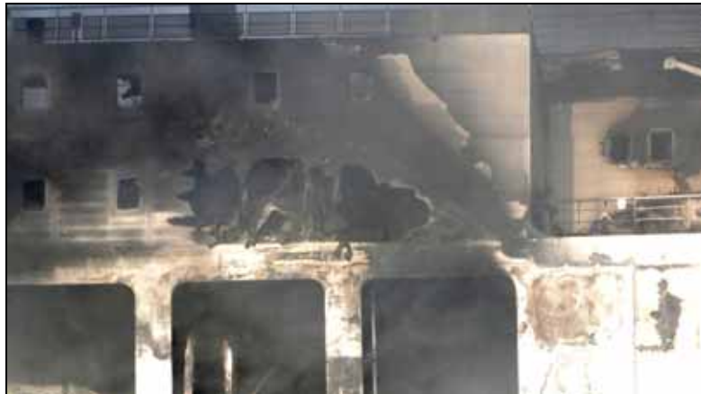
Figure 115: Hole in the outer wall on deck 7, taken on 9 October 2010 at 1456
