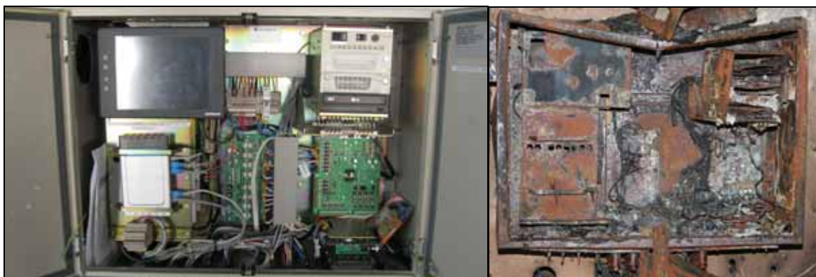
Figure 122: VDR main unit in its original condition (model for comparison) and after the fire
