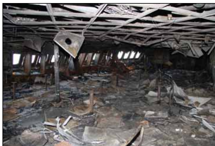
Figure 21: Burned-out bar area
