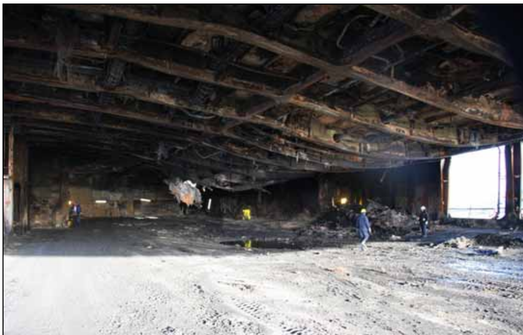
Figure 33: Partly cleared deck 6 with debris at the observed source of the fire
