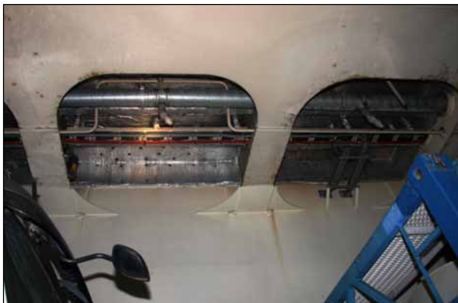
Figure 58: A-60 insulation on deck 2
