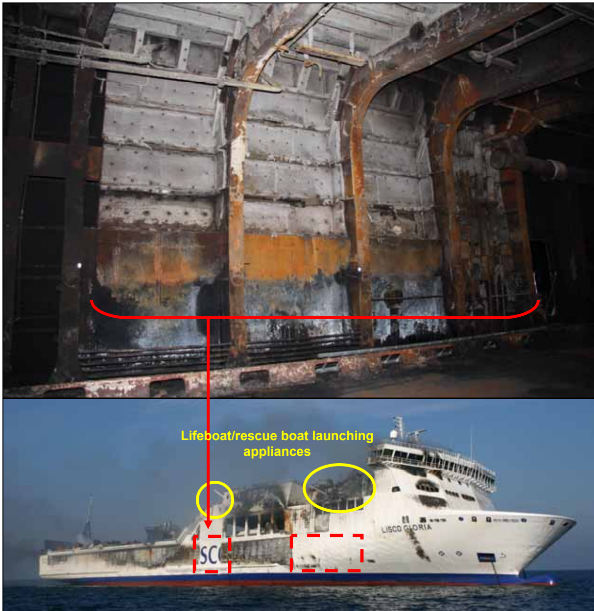
Figure 62: Reinforced insulation in the area of the life-saving equipment
