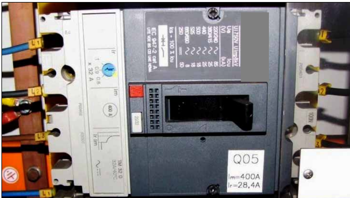
Figure 91: Circuit breaker, close up
