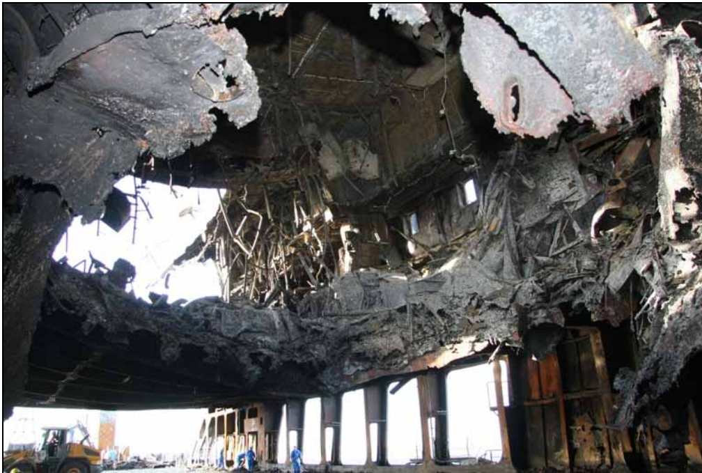
Figure 17: Fire funnel opening between deck 6 and the accommodation decks above
