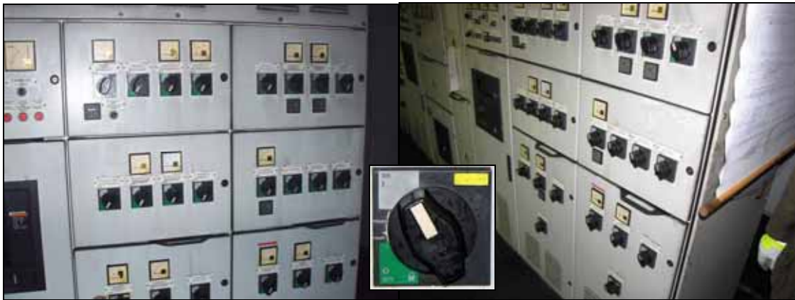
Figure 43: Part of the main switchboard on 11 October 2010 (left) and on 25 October 2010 (right)
