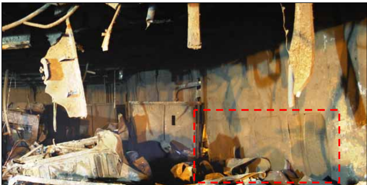
Figure 76: Ventilation ducts on deck 4 – starboard side
