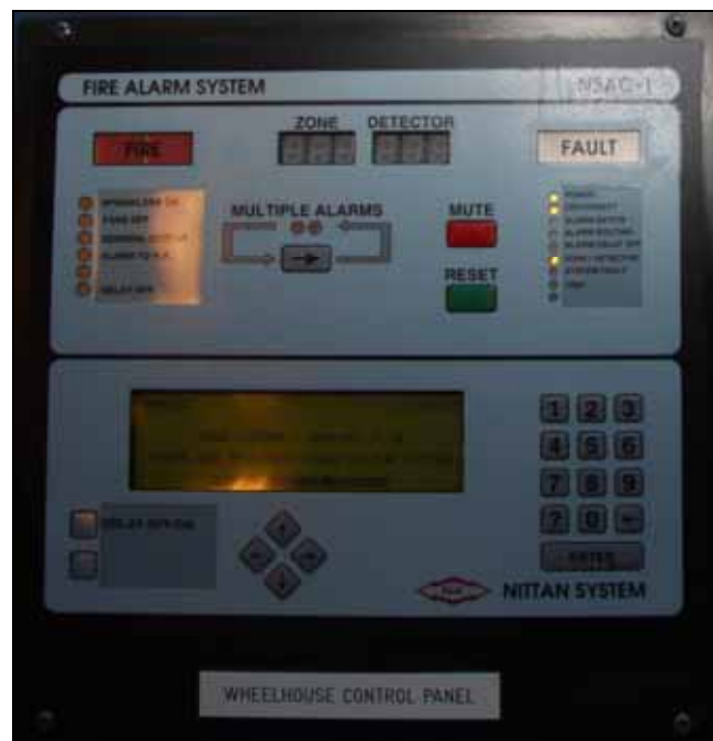
Figure 68: Control panel of the identical fire alarm and detection system on the sister vessel, DANA SIRENA
