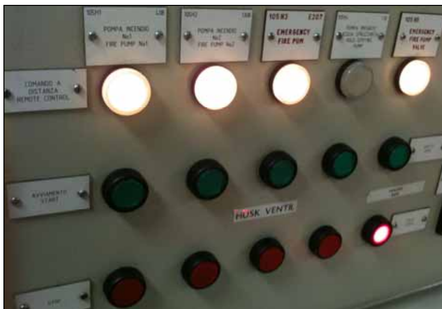
Figure 84: Control panel for the fire and drencher pumps in the engine control room of the DANA SIRENA when the valve setting on the switchboard for the drencher pump has been changed
