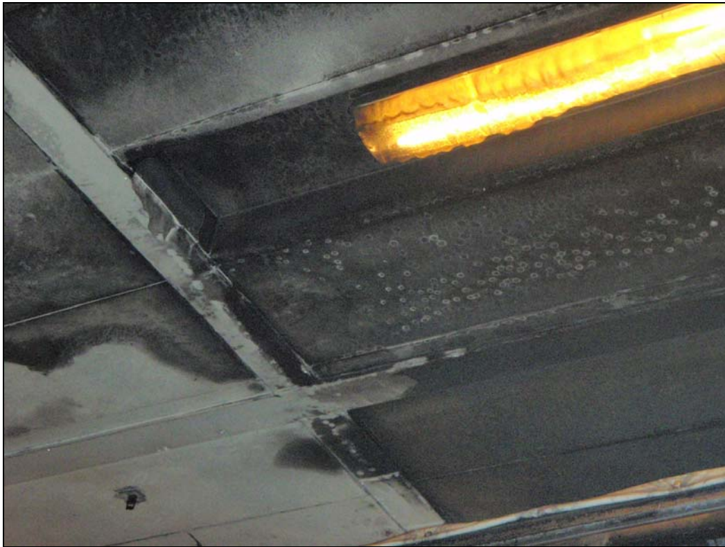
Figure 5: Close-up of the scorch marks on the ceiling
