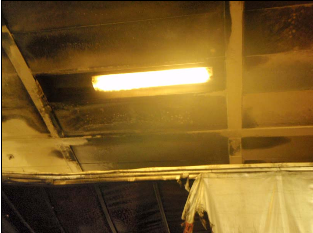
Figure 4: Scorch marks on the ceiling above the scene of the fire
