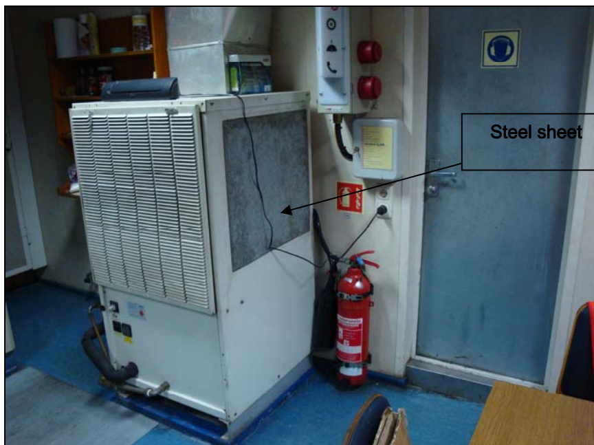
Figure 4: Ventilation fan with closed steel sheet
