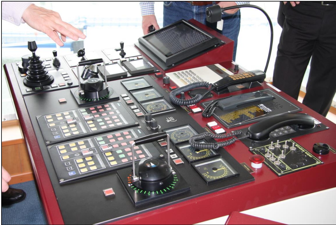
Figure 18: Control position in the port wing
