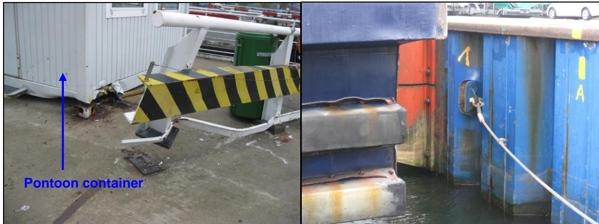
Figure 16: Damaged guardrail and damaged sheet piling at the pier
