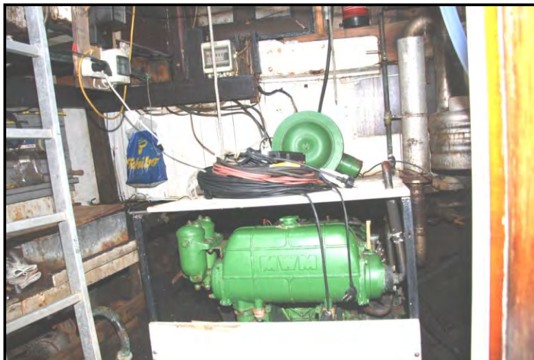
Figure 20: Shore electric power supply
