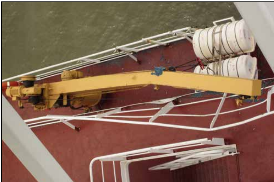
Figure 7: Damage to the superstructure (provision crane) of the CCNI RIMAC
