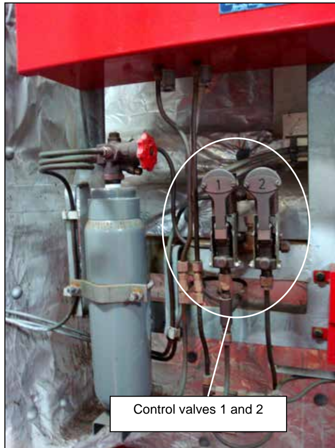
Figure 11: MSC ALESSIA – control valves 1 and 2 in the normal position (closed)
