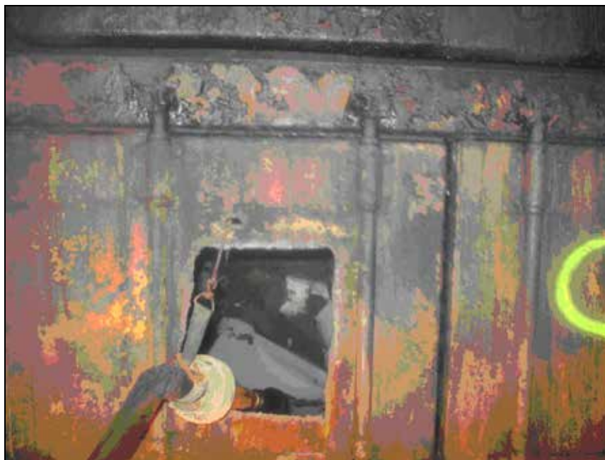
Figure 27: Cut open container in cargo hold 7 with suspended nozzle
