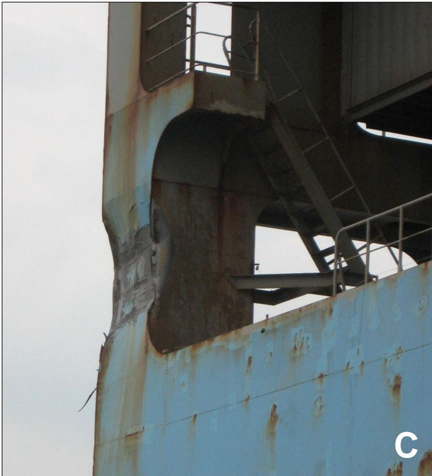
Figure 21: Damage to the cell guide foundation on the starboard side of the aft edge (close-up)
