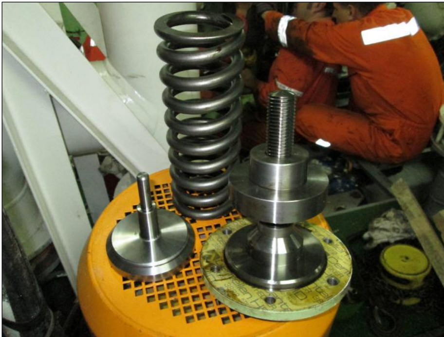
Figure 34: Pump safety valve after disassembly
