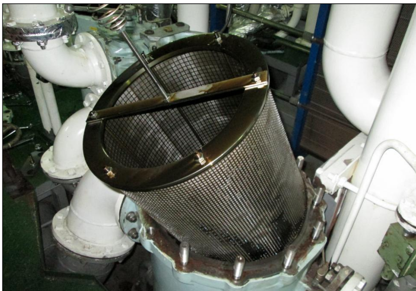
Figure 30: Suction filter on the standby pump
