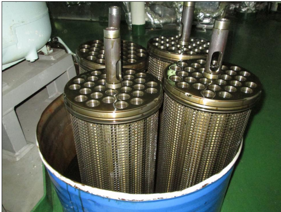
Figure 31: Automatic backwash filter
