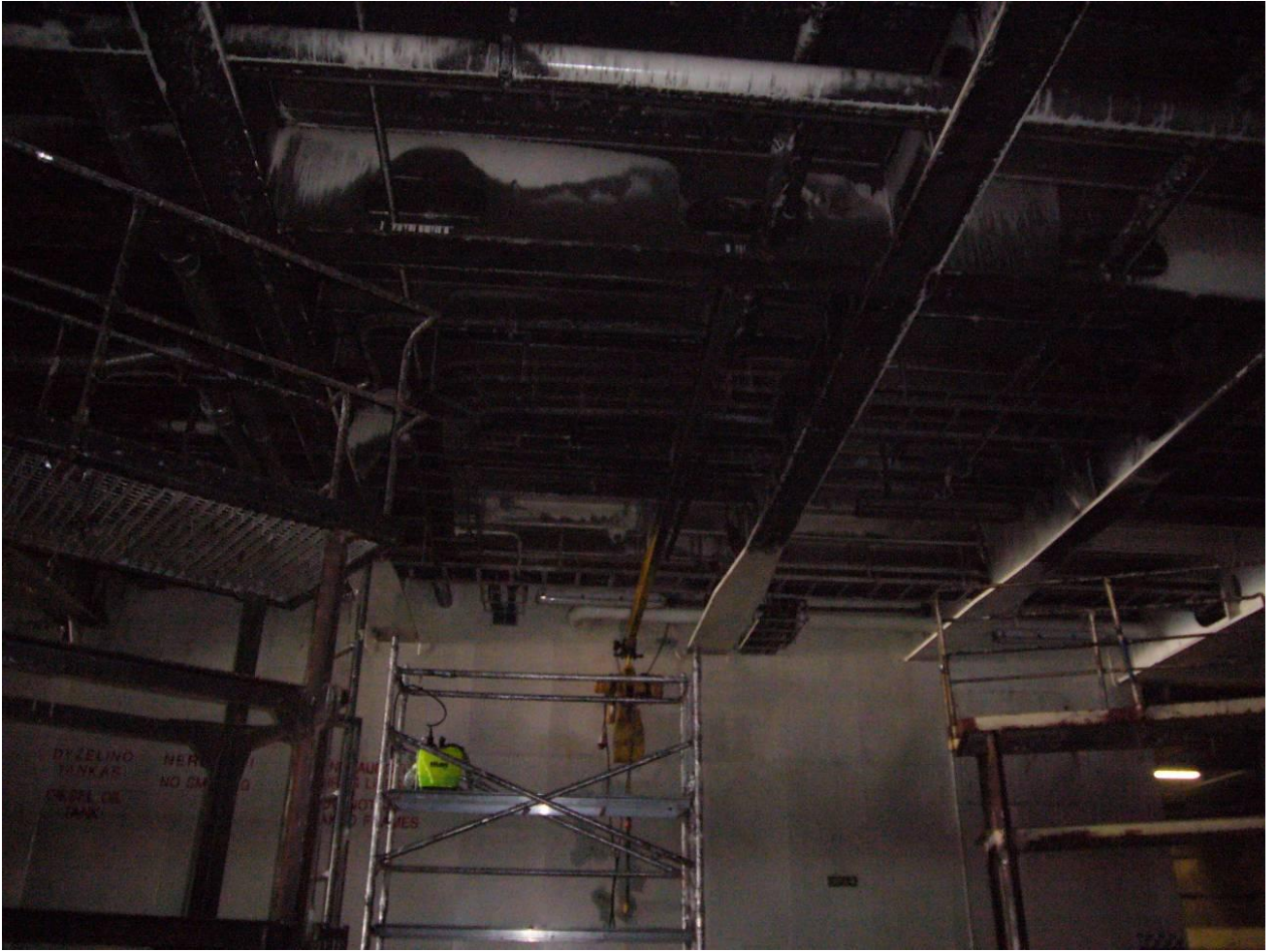
Figure 5: Sooty deck roof
