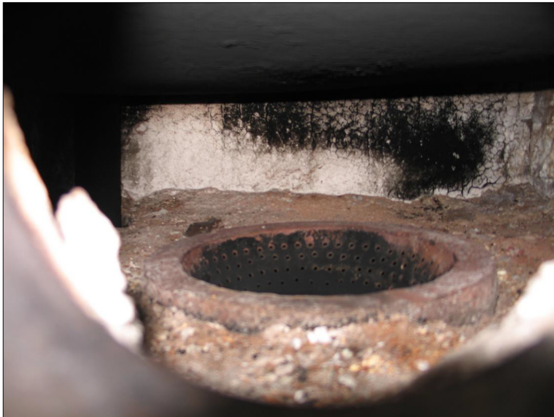
Figure 10: Cup burner below the tank
