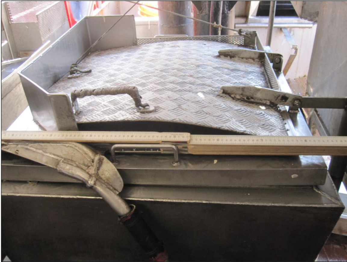
Figure 18: Buckled boiler lid
