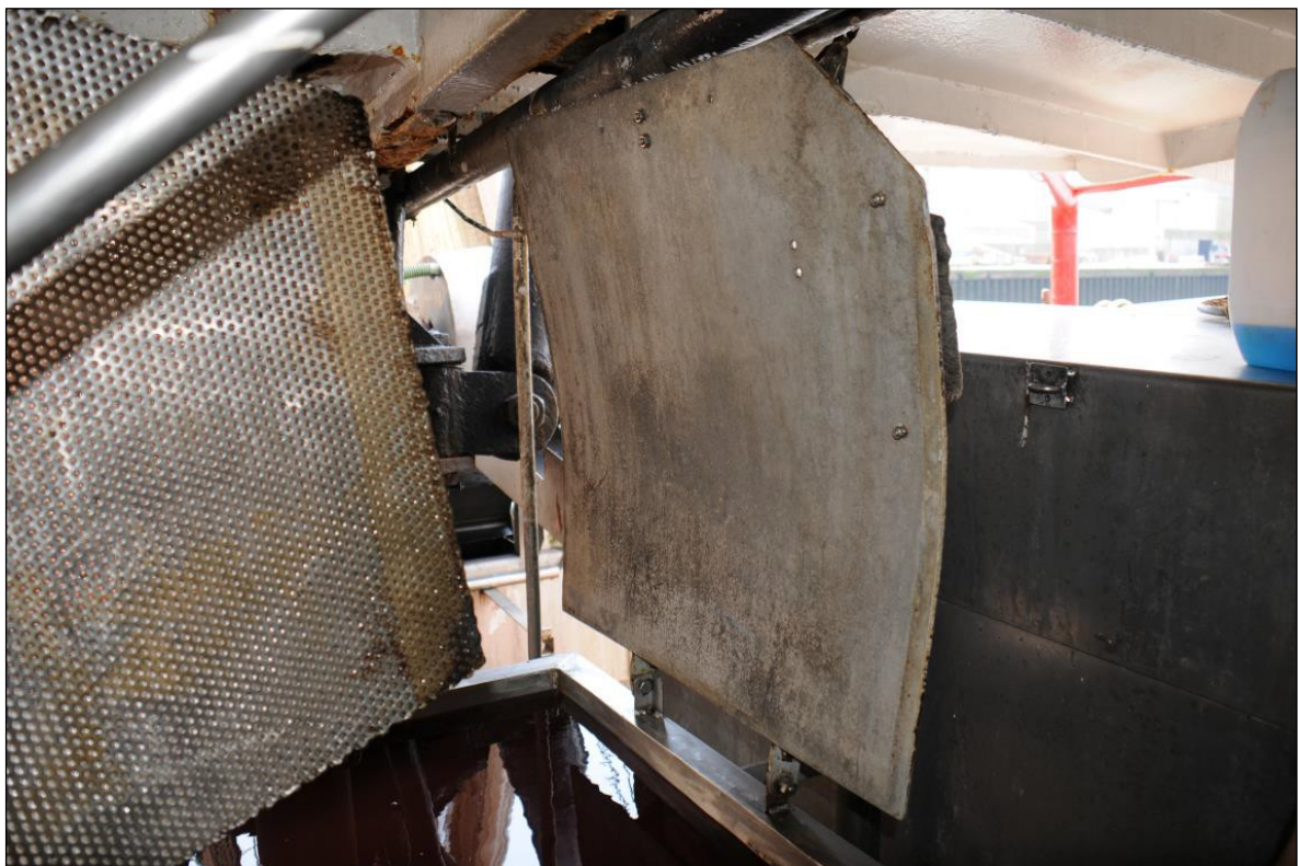
Figure 17: Deck structure struck by lid
