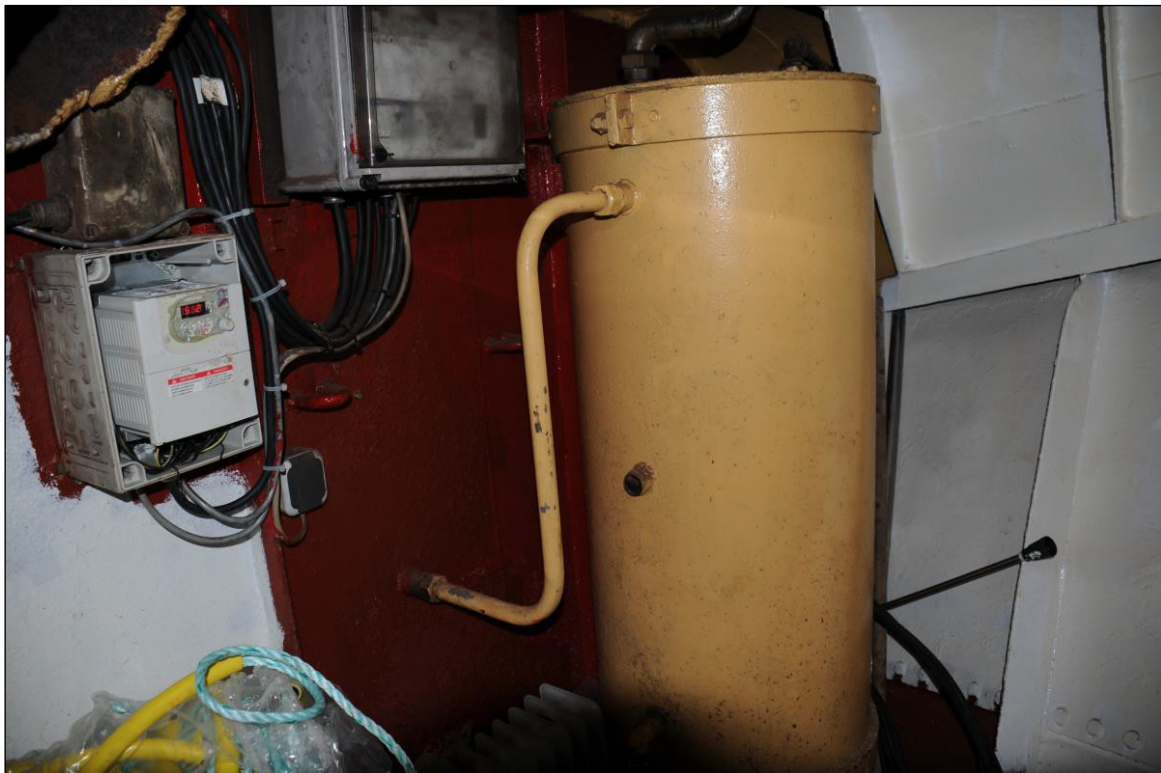
Figure 4: Diesel tank beneath the forecastle
