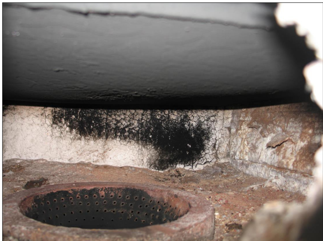
Figure 11: Insulated interior of the combustion chamber
