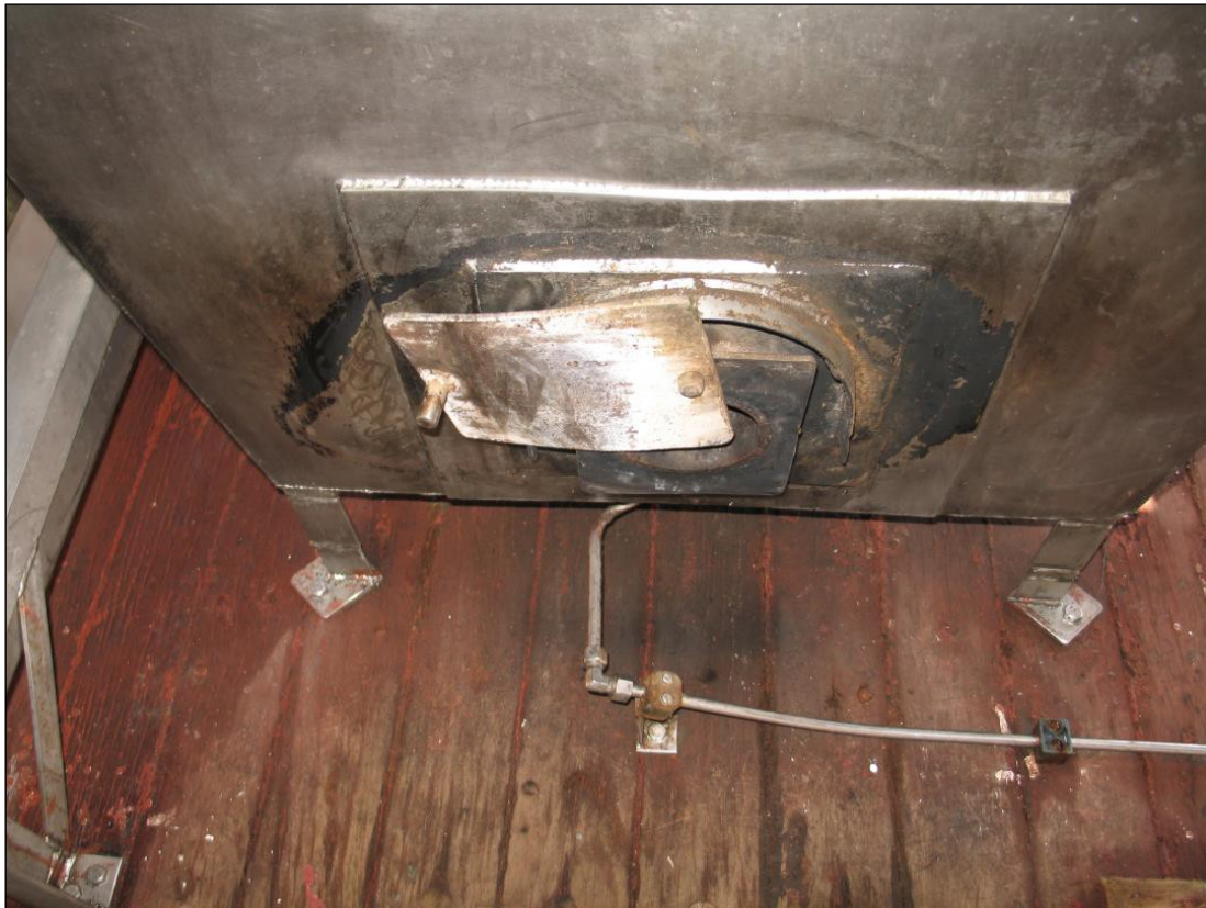
Figure 8: Fuel line to the boiler
