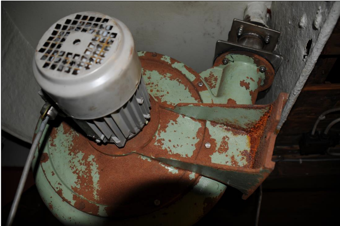
Figure 16: Blower below deck
