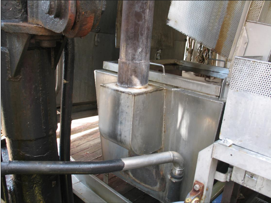
Figure 12: Waste gas/exhaust ventilation duct
