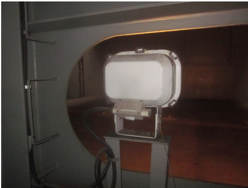
Figure 7: Central main floodlight at the transverse passageway
