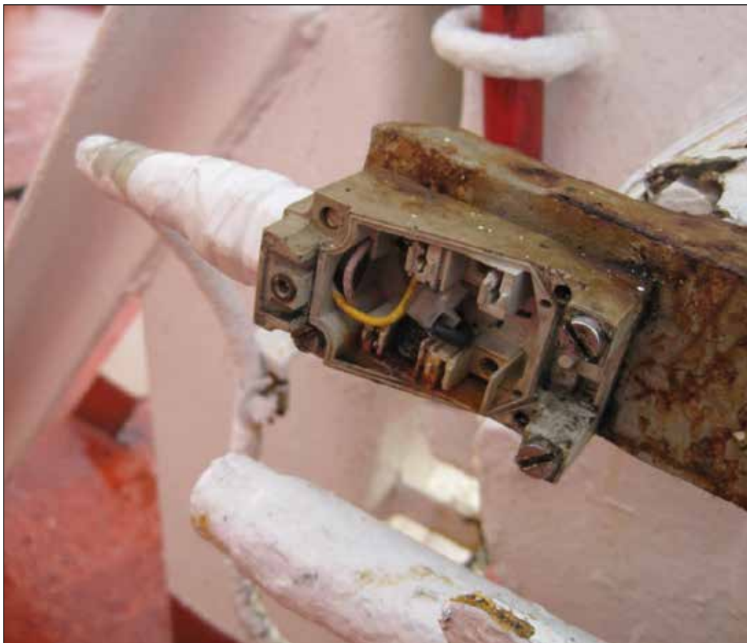
Figure 17: Corroded switch on the winch
