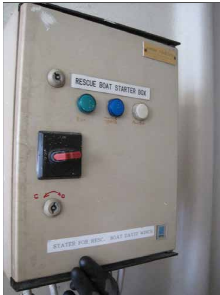
Figure 18: Control panel for the electrics on the poop deck
