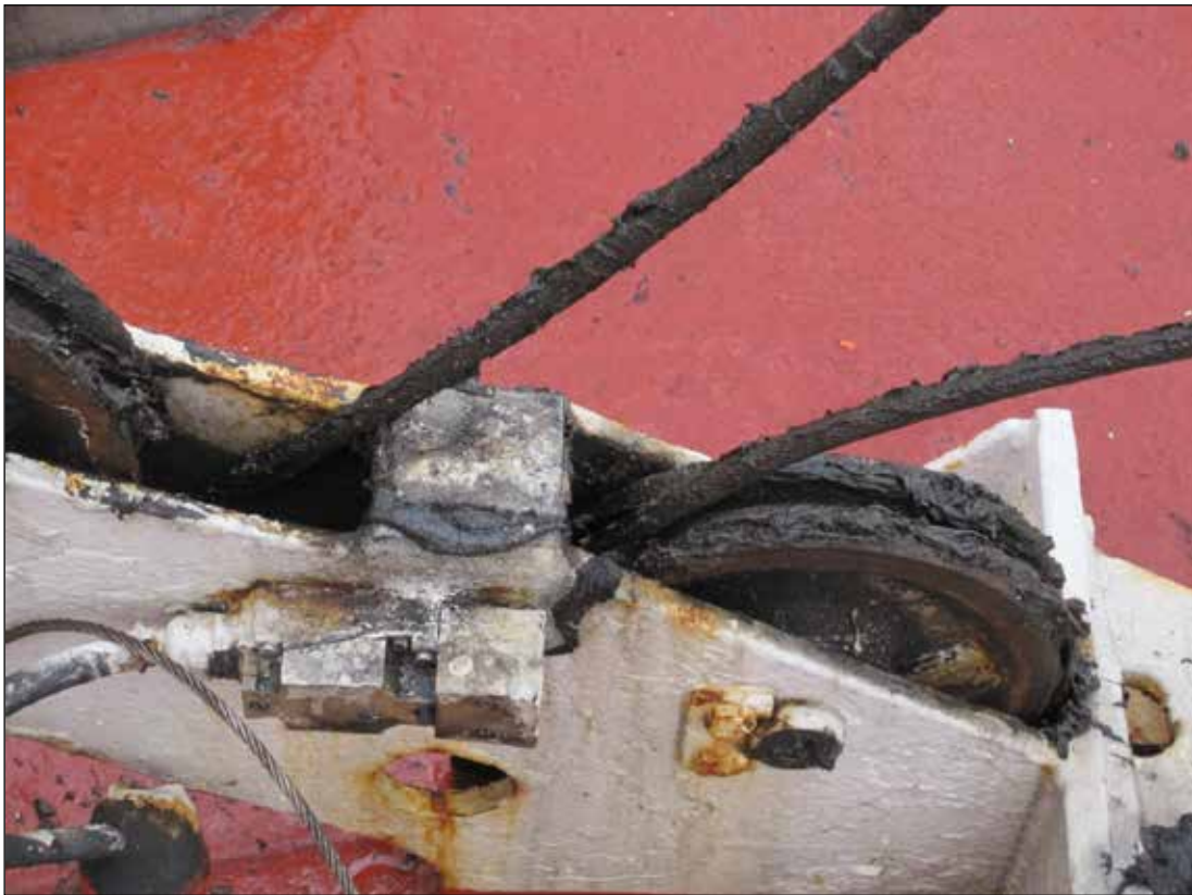
Figure 14: Grease on cable, guide pulley, and in the housing
