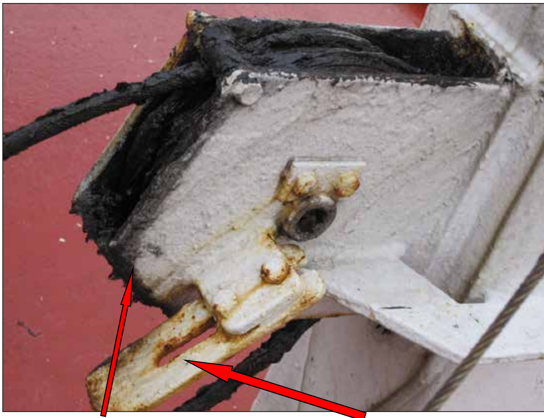
Figure 31: Limit switch's companion part with the support surface for the davit's limit next to it
