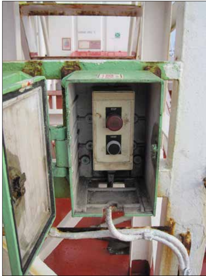
Figure 19: Electrical hoist/emergency shutdown pushbutton next to the davit system
