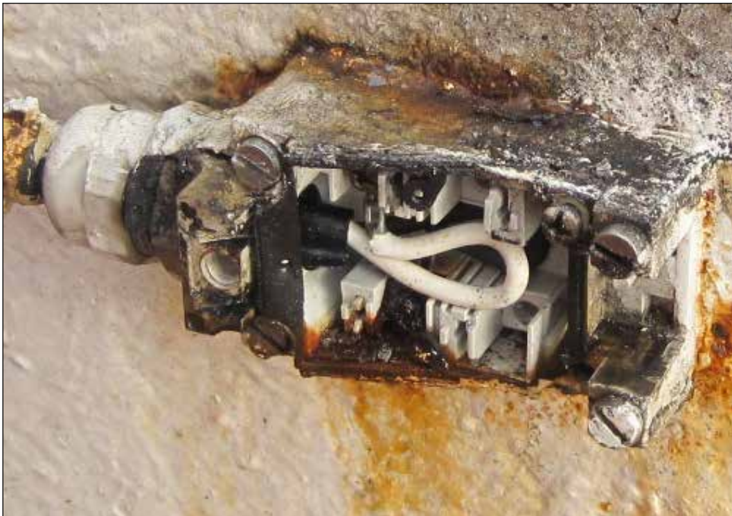
Figure 16: Corroded limit switch with defective seal
