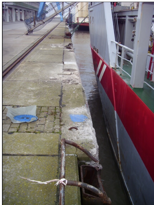
Figure 8: Damage to the pier
