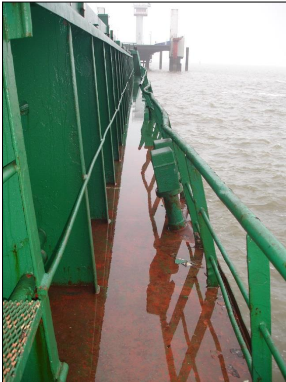
Figure 4: Guard rail damage (BIMI)
