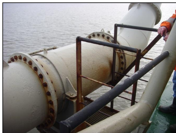
Figure 7: Drain pipe (BARENT ZANEN)
