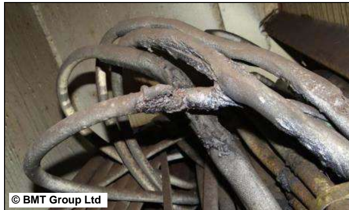
Figure 66: Example of charred cable insulation (1) 39
