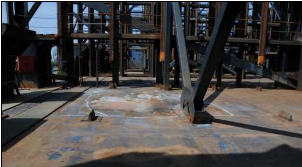
Figure 56: Warped deck and fire damage in the area of bay 26
