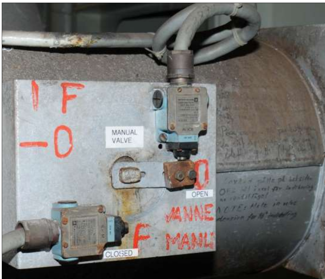
Figure 34: Main tank valve with handwritten operating instructions
