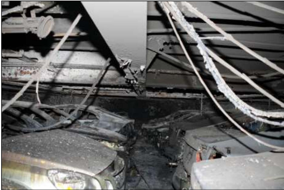
Figure 47: Thermal stress on the deck's ceiling
