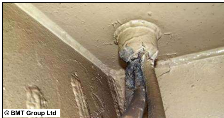
Figure 68: Example of charred cable insulation (3) 41
