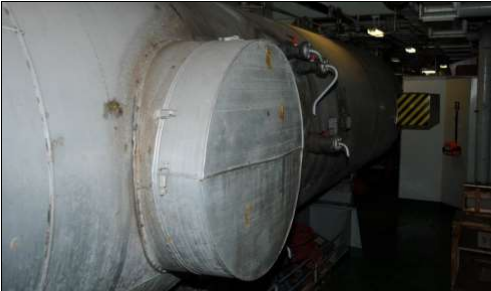
Figure 16: CO 2 low-pressure tank
