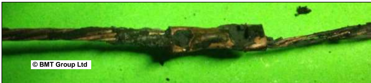
Figure 65: Cable splice with inconsistencies in respect of diameter and number of conductors 38
