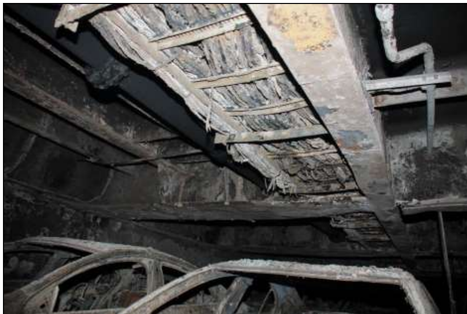
Figure 54: Destroyed cable routing and deformed girders beneath the ceiling
