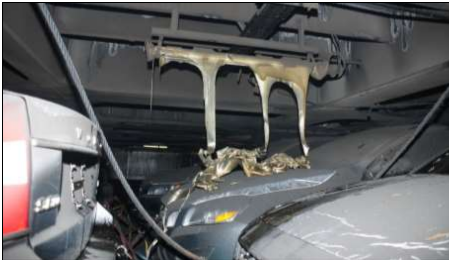
Figure 52: Plastic casing of a ceiling light melted by heat radiation
