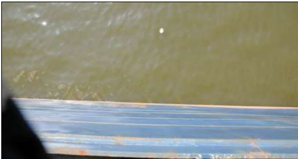
Figure 58: No thermally induced damage to the hull wall in the area of bay 26 (port side)
