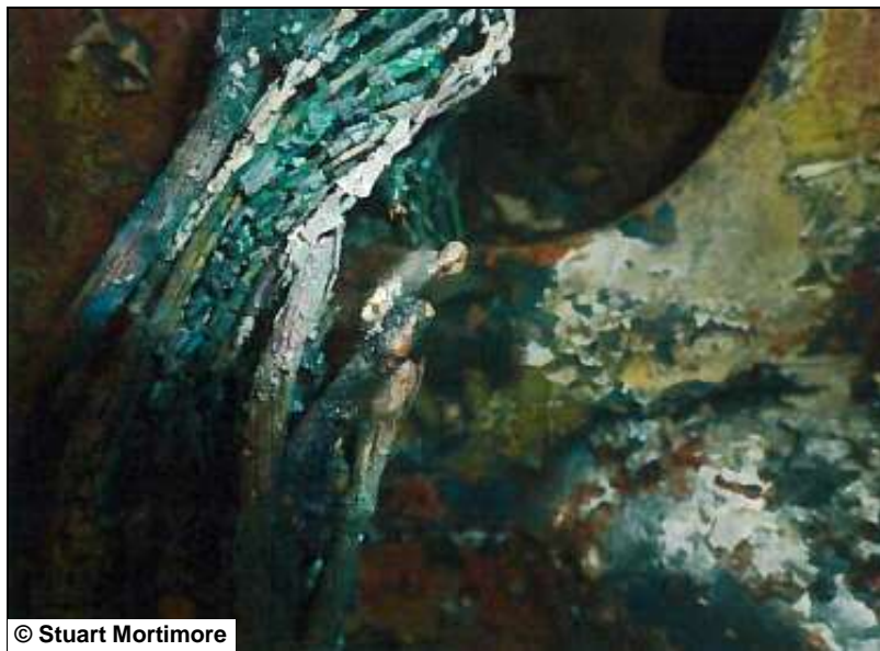
Figure 102: Example of arcing activity caused by electric current (1) 75
