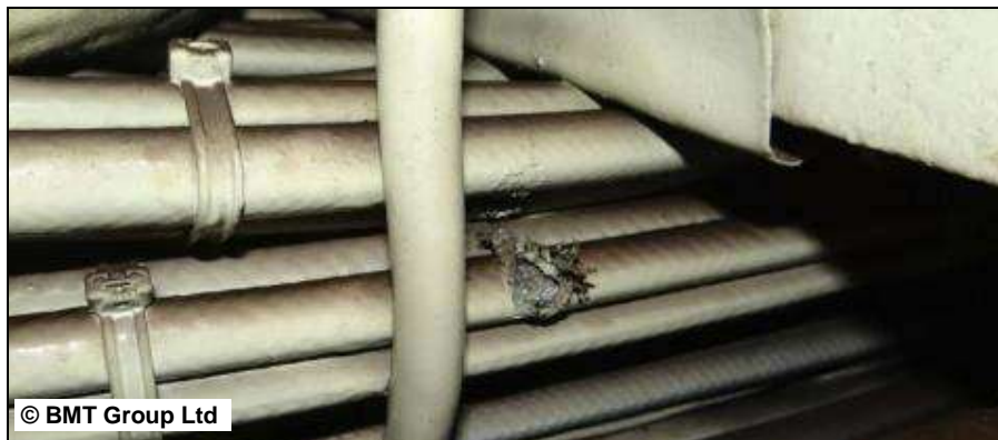
Figure 67: Example of charred cable insulation (2) 40
