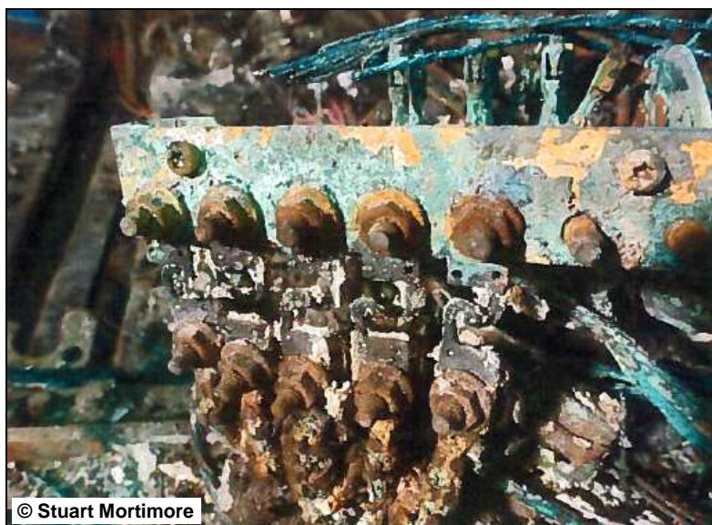
Figure 104: Close-up of the fuse box in the engine compartment of vehicle 5 A 77
