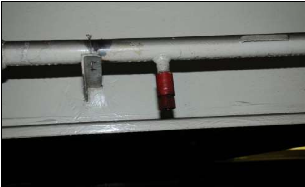
Figure 17: CO 2 system line with gas nozzle in the cargo hold
