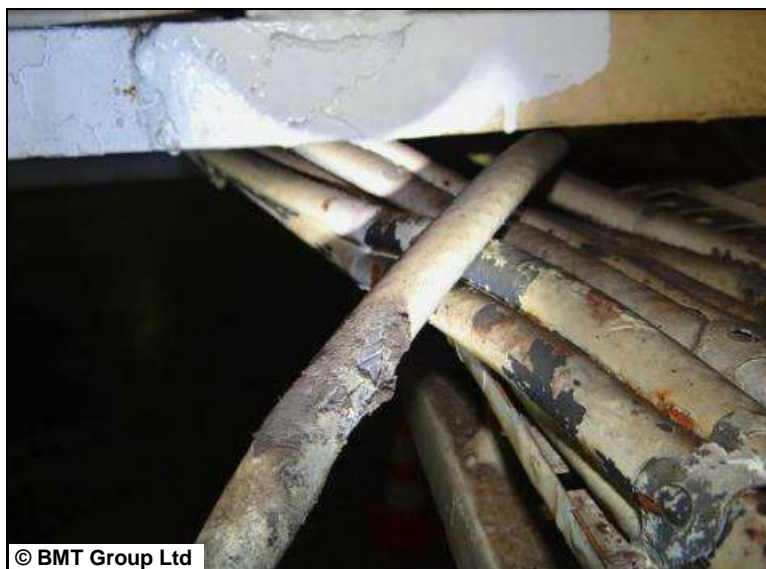
Figure 72: Example of cable insulation damaged by welding operations (2) 45
