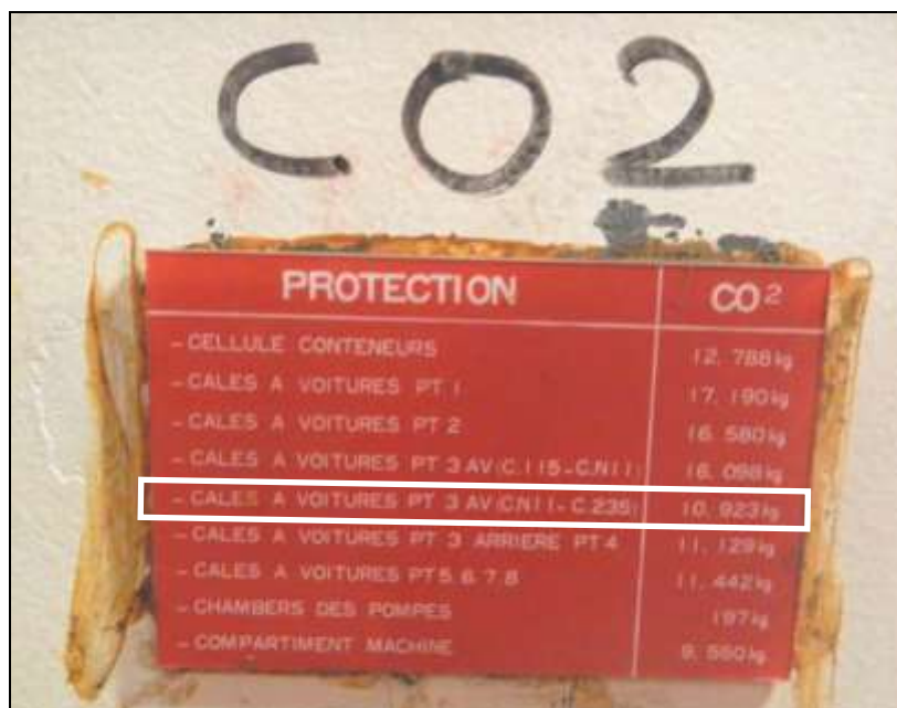
Figure 28: Overview of the CO 2 flood quantities (CO 2 control room)
