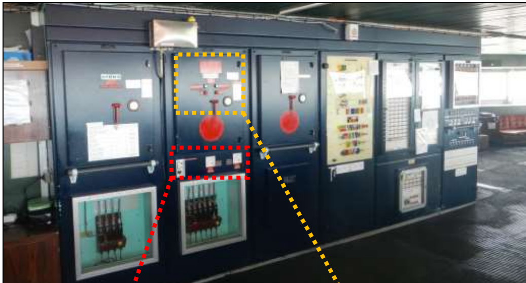
Figure 18: Complete alarm and control panel on the bridge for the extinguishing system
