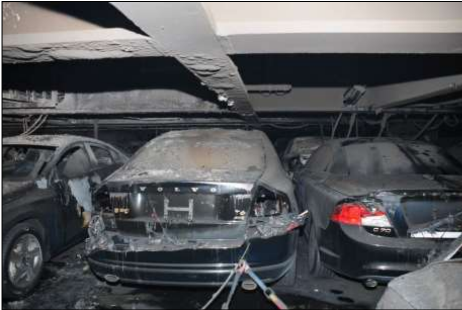
Figure 51: Destroyed plastic parts (in this case the rear lights) on the vehicles
