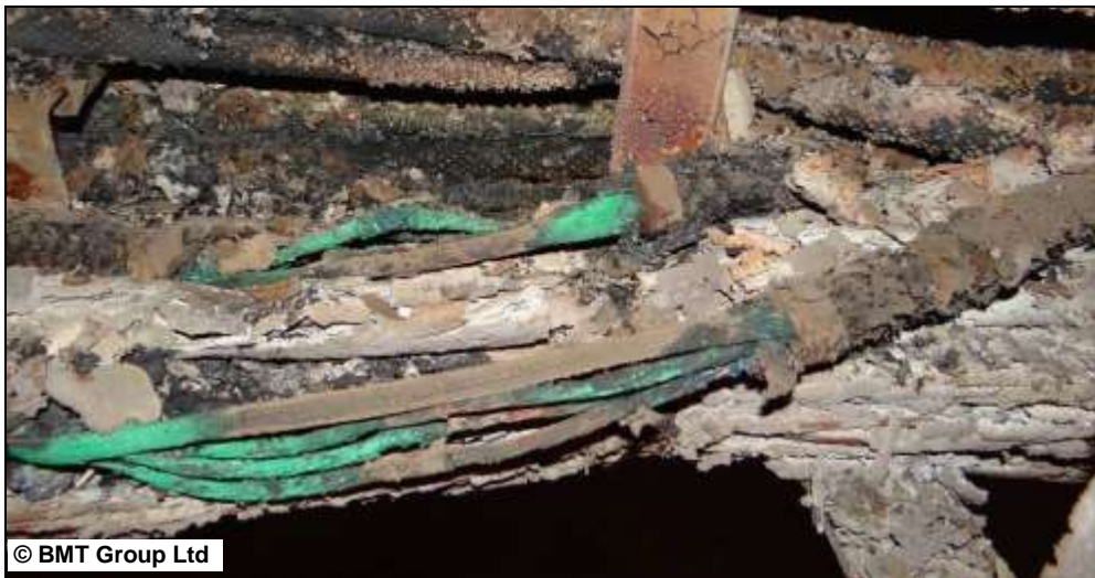
Figure 74: Example of conspicuous signs of corrosion in the wiring 47
