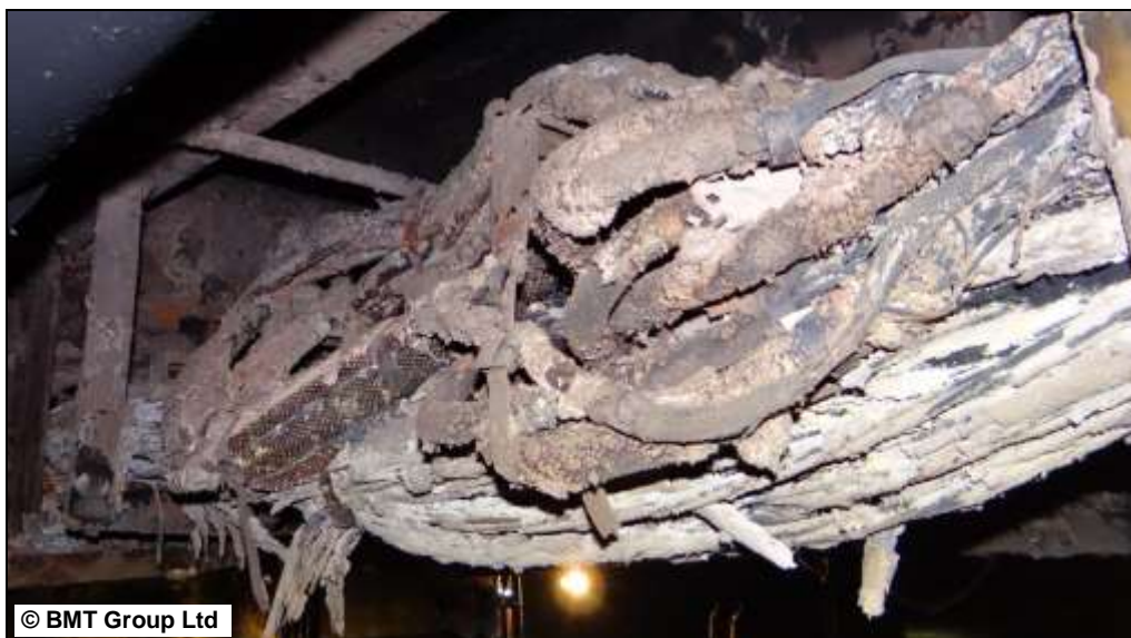
Figure 62: Cable splices on the ceiling of vehicle deck 3 B (close-up) 35
