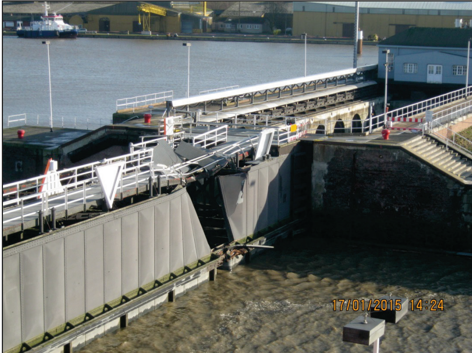
Figure 20: Damage to the lock gate
