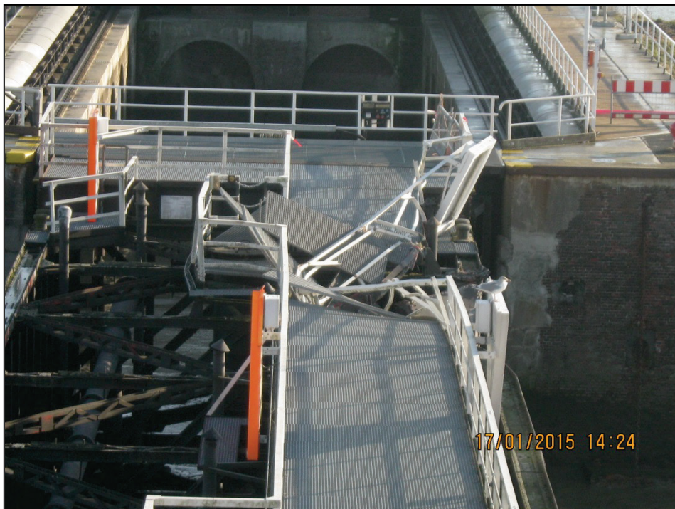
Figure 21: Damage to the lock gate's walkway
