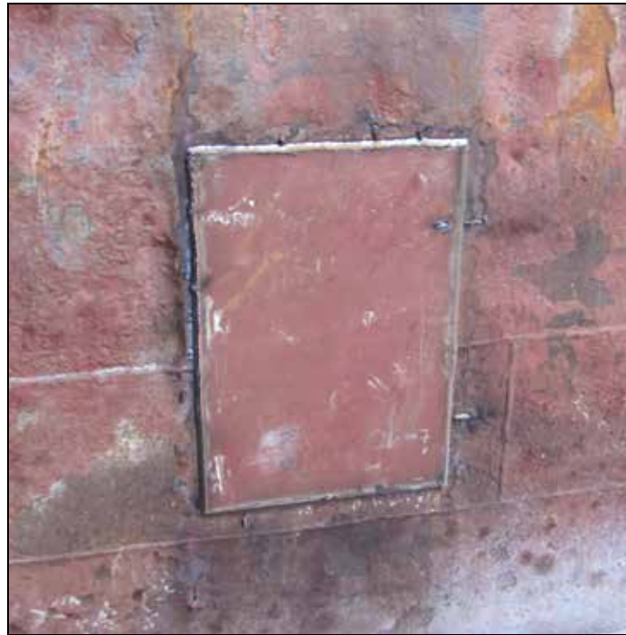
Figure 44: Manhole cover welded closed using a steel plate
