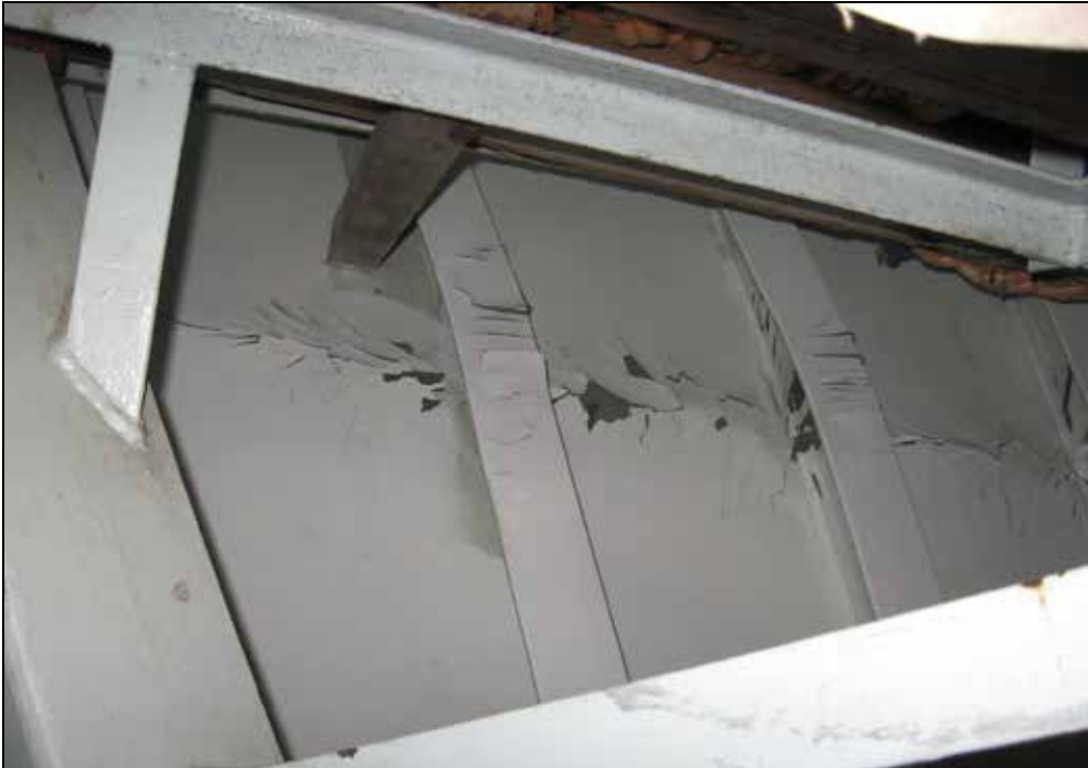
Figure 7: Damage to CORAL IVORY's stem (view inside)
