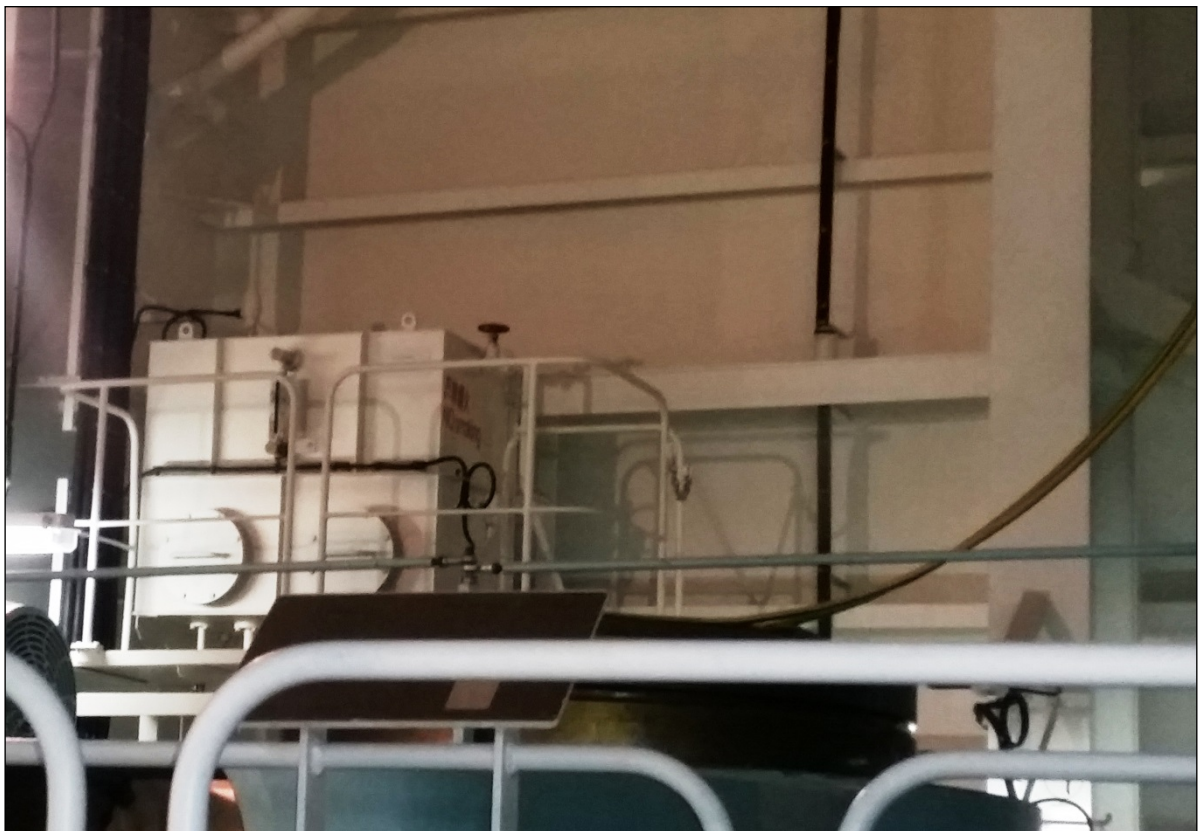
Figure 18: Hydraulic fluid tank
