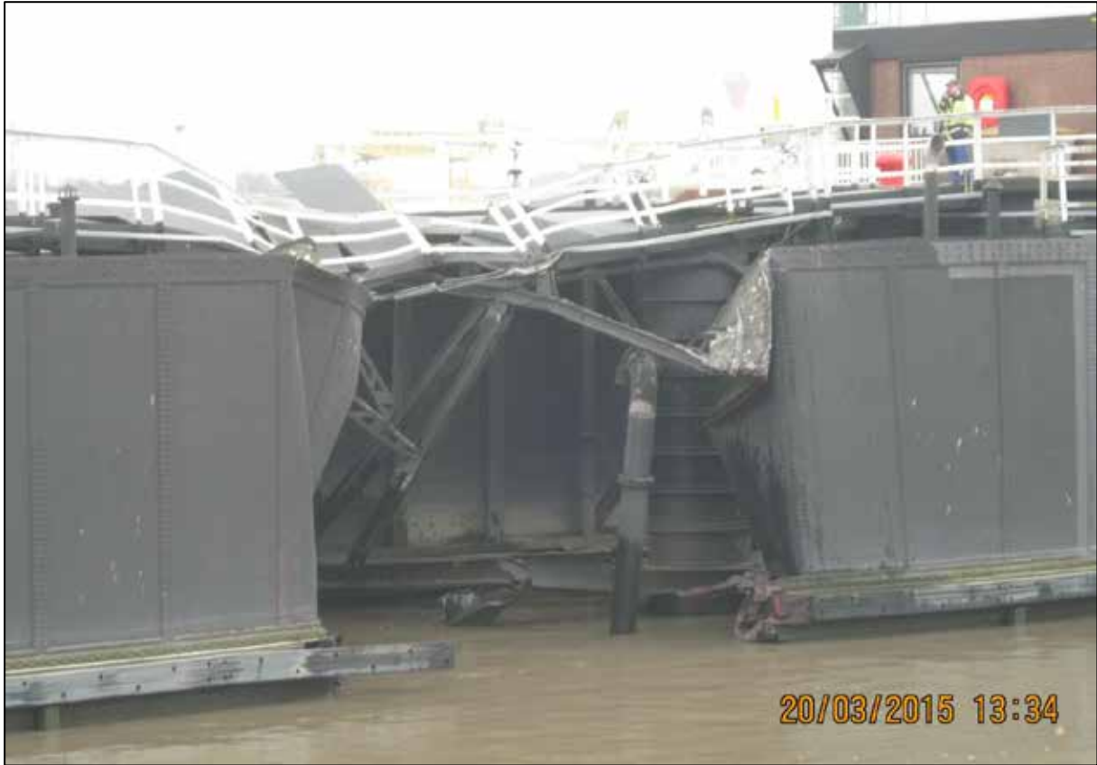
Figure 5: Damage to the lock gate
