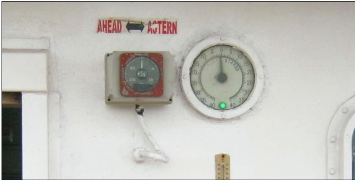
Figure 14: Indicators in the starboard wing
