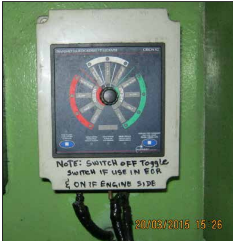
Figure 12: Engine order telegraph at the engine's control stand
