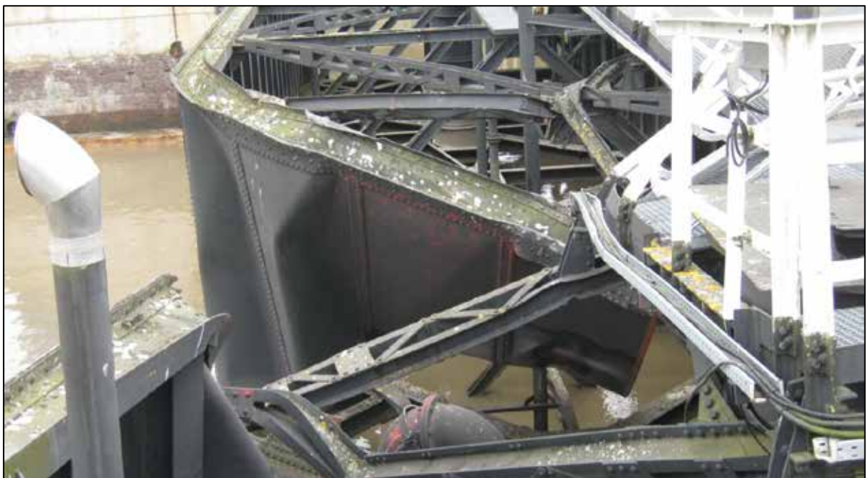
Figure 6: Damage to the lock gate
