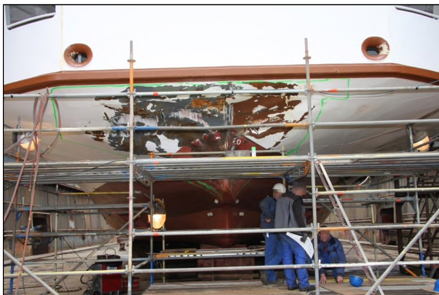
Figure 15: Damage to the ferry's bow section (front view)
