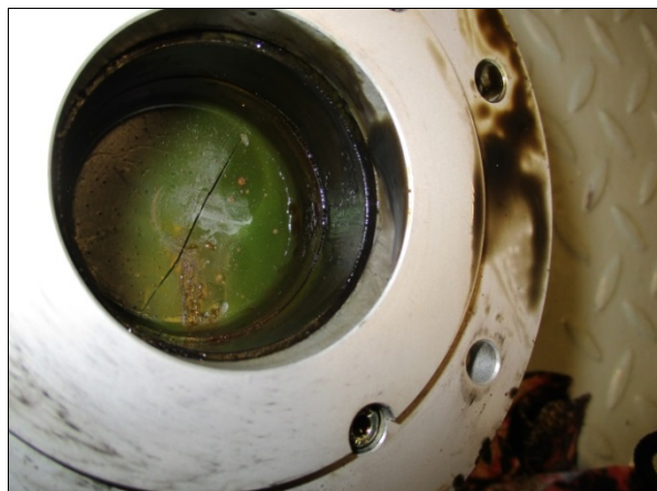
Figure 7: Crack in Hall generator
