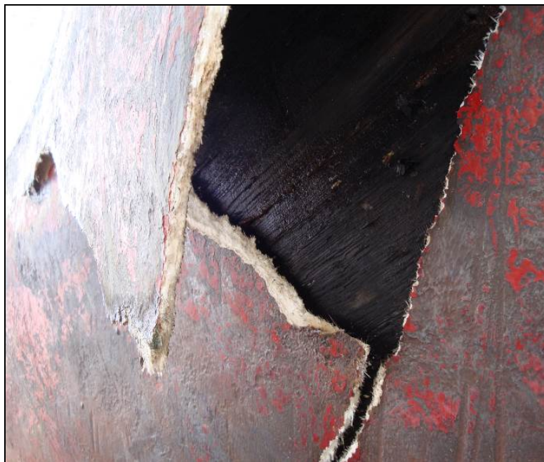
Figure 16: Cracks in the GRP coating (close-up)
