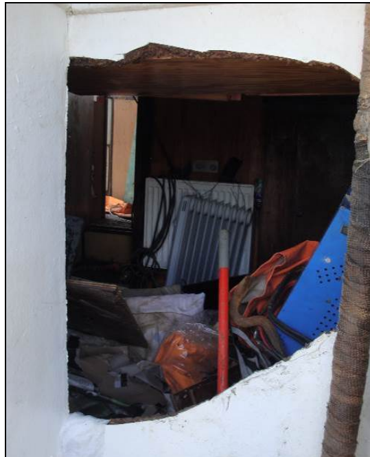
Figure 21: Hole in the partition wall between the companionway and skipper's berth
