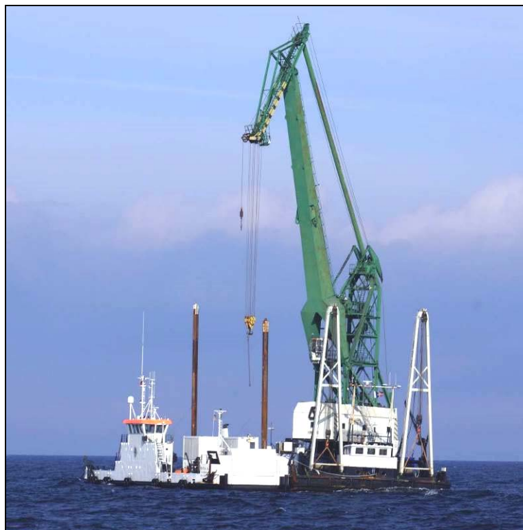
Figure 4: Floating crane SANNE A and multipurpose ship MIRA A (preparing for the salvage operation)
