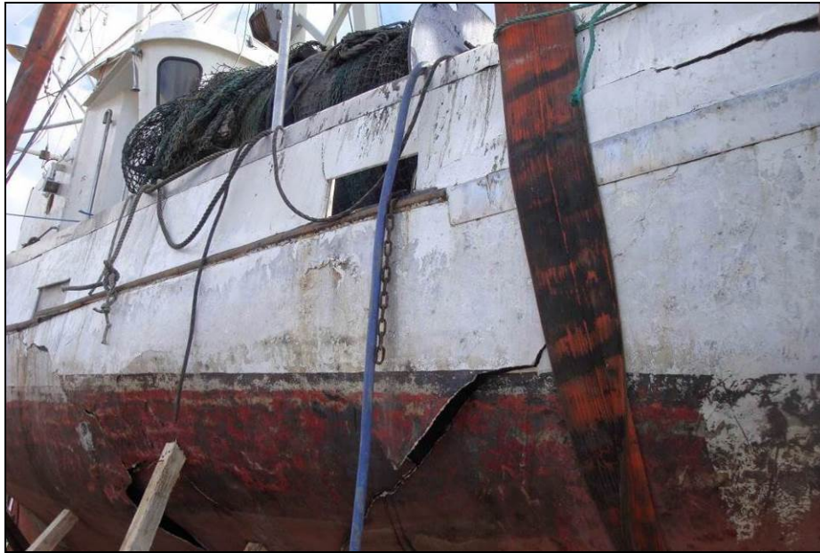
Figure 15: Cracks in the GRP coating
