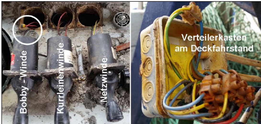
Figure 101: Electrical winch control
