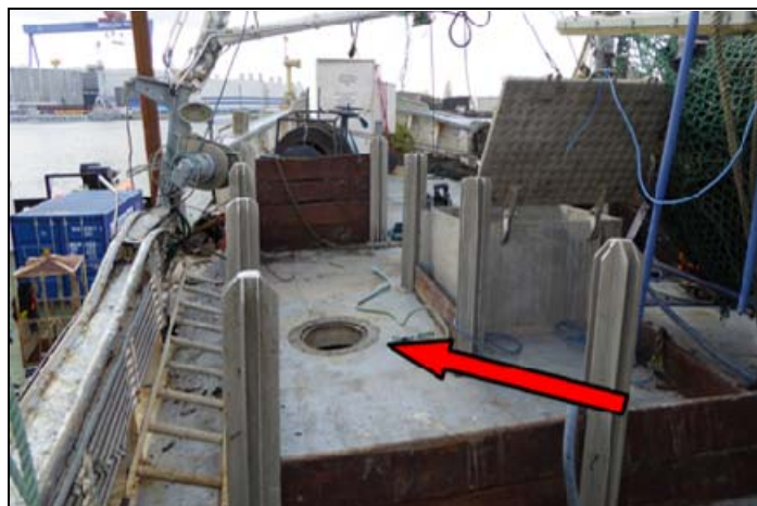
Figure 106: Absent bolting between the deck and fish hold
