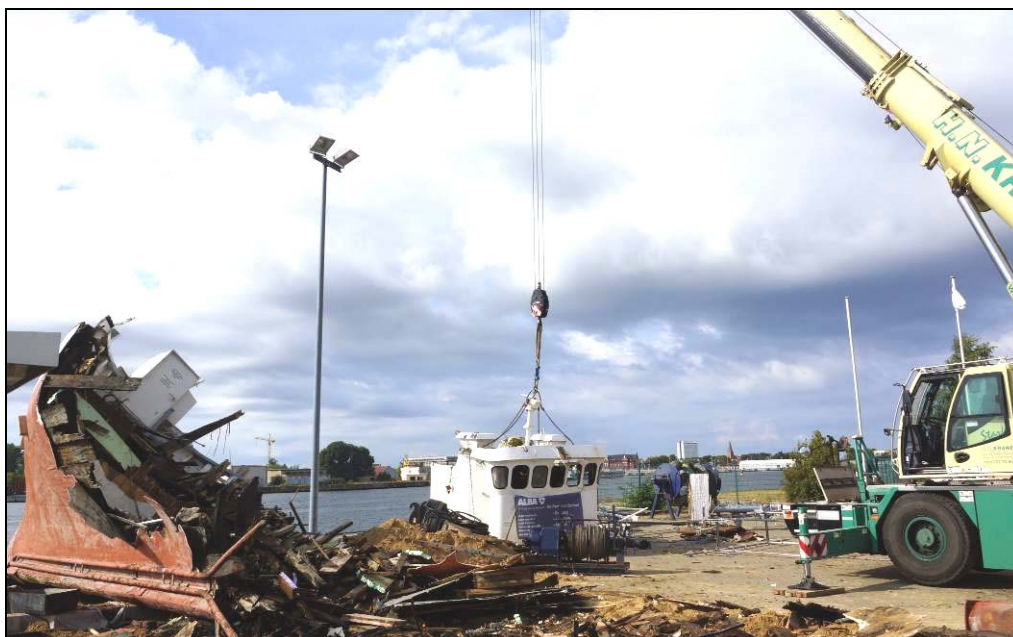
Figure 11: Determination of individual masses when the fishing vessel was dismantled (above the wheelhouse) in September 2016
