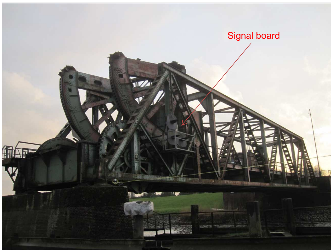
Figure 18: Northerly passage with destroyed bascule and signal board
