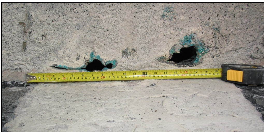
Figure 31: Rust penetration at the bottom of the cargo hold 3 to cargo hold 2 bulkhead
