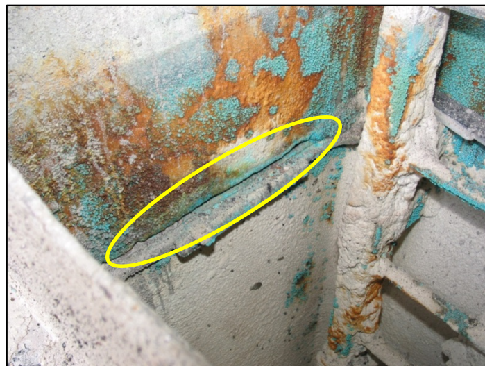
Figure 34: More rust penetration in the hold ladder's trunk Cargo hold 3, forward edge of the tween deck, port side. View to the left from the entrance toward void space B (see Figure 35)
