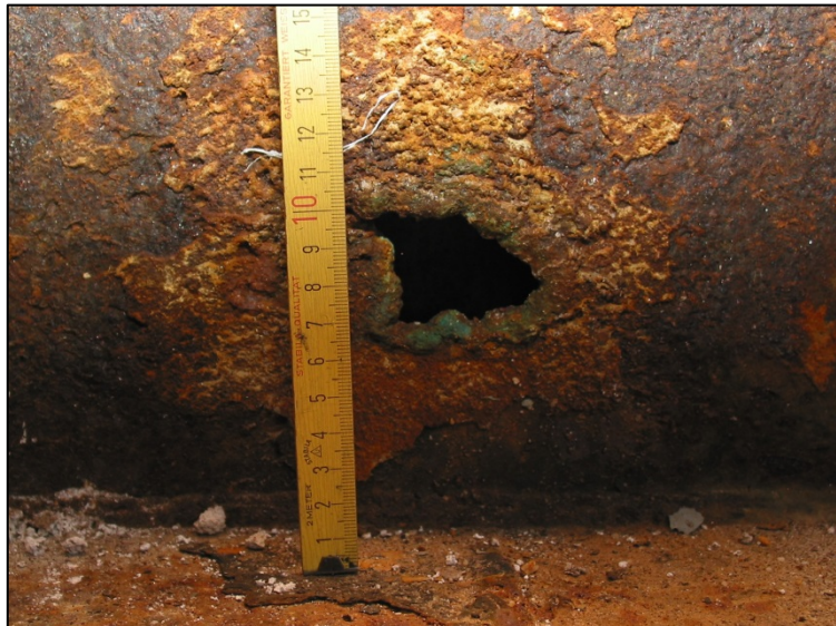
Figure 54: Close-up to Figure 49, hole C
