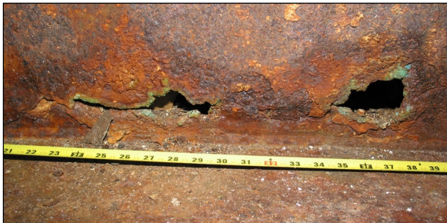
Figure 51: Close-up to figure 49, holes A and B
