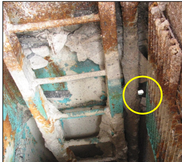
Figure 33: Rust penetration in the hold ladder's trunk on the port side (here the cargo hold 3 to cargo hold 2 bulkhead)
