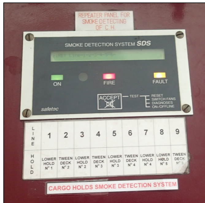
Figure 9: Smoke detection system's display on the bridge
