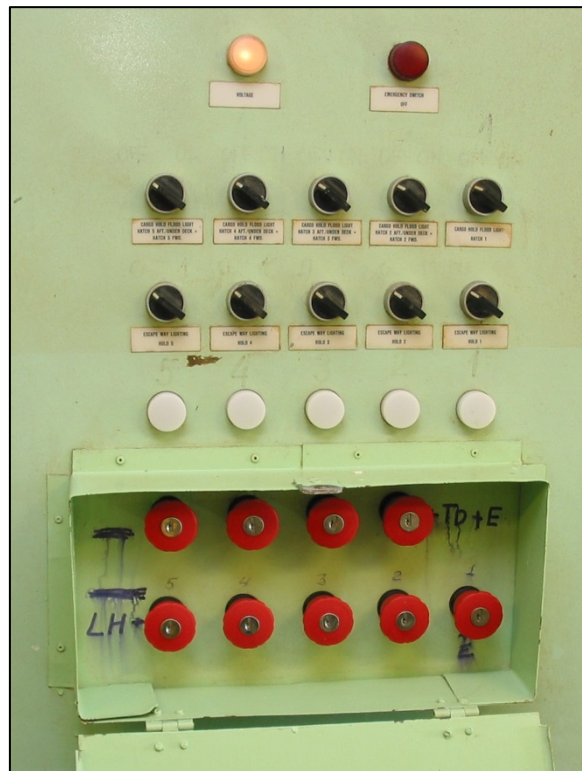
Figure 24: Control panel for the cargo hold lighting with cover open
