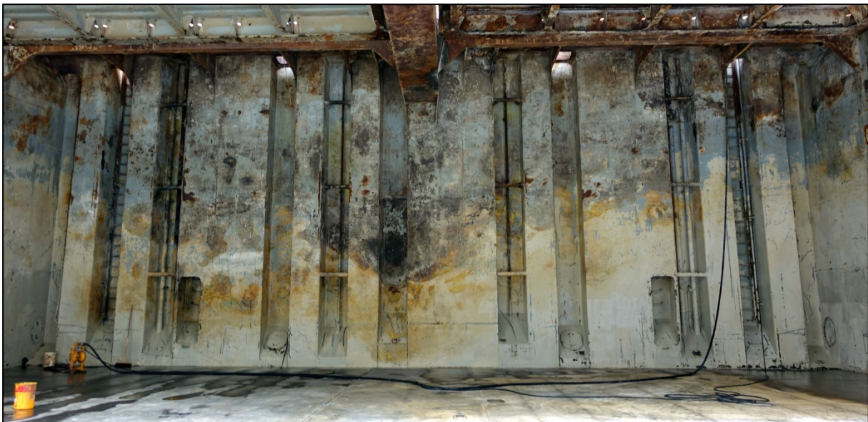
Figure 42: Cargo hold 3's lower hold, aft bulkhead edge Traces of intense heat on the aft transverse bulkhead from a height of 2.2 m
