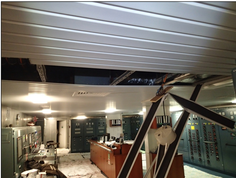
Figure 8: ECR with detached ceiling lining
