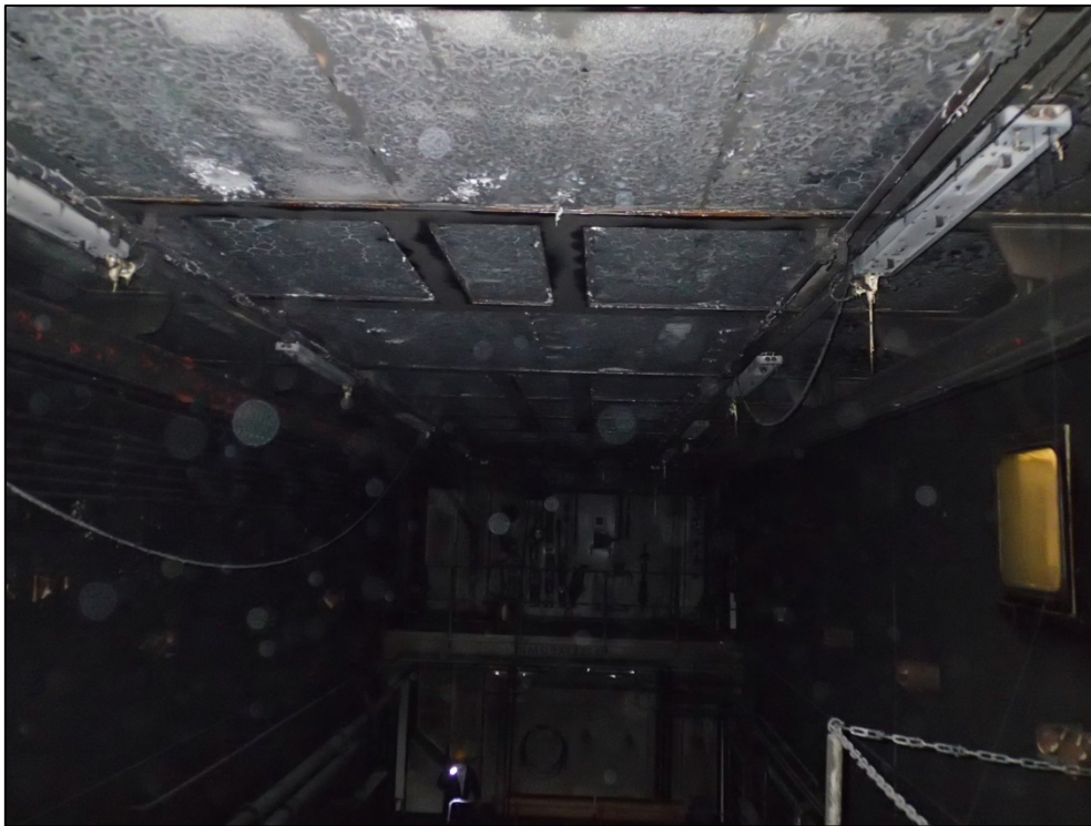
Figure 7: Traces of fire in the engine room
