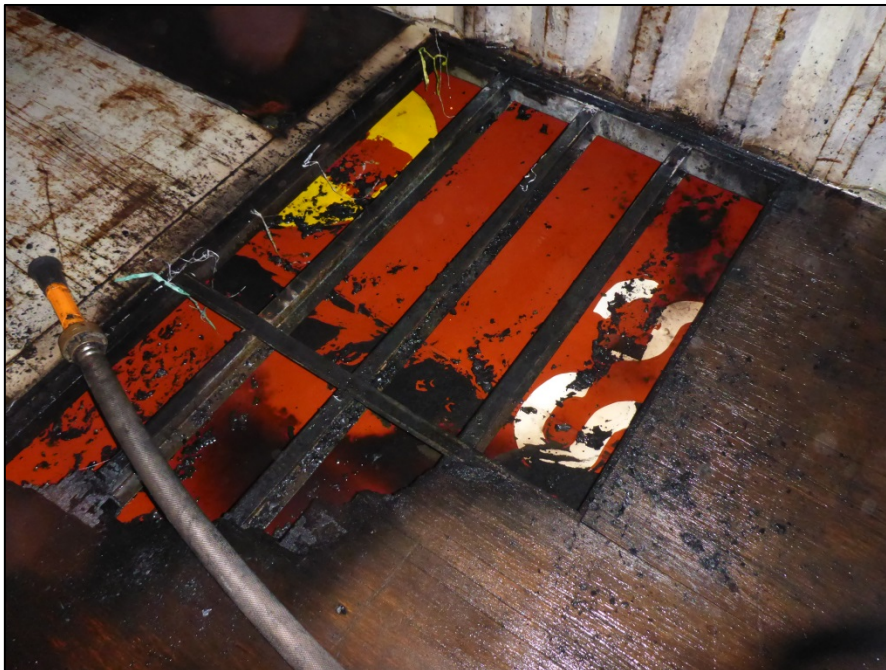
Figure 20: Container bottom burnt through
