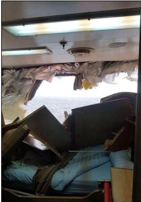
Figure 13: Damage to the outer wall of a cabin
