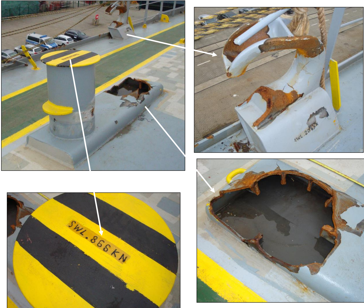
Figure 11: Close-ups of the destroyed bollard and broken hawsehole
