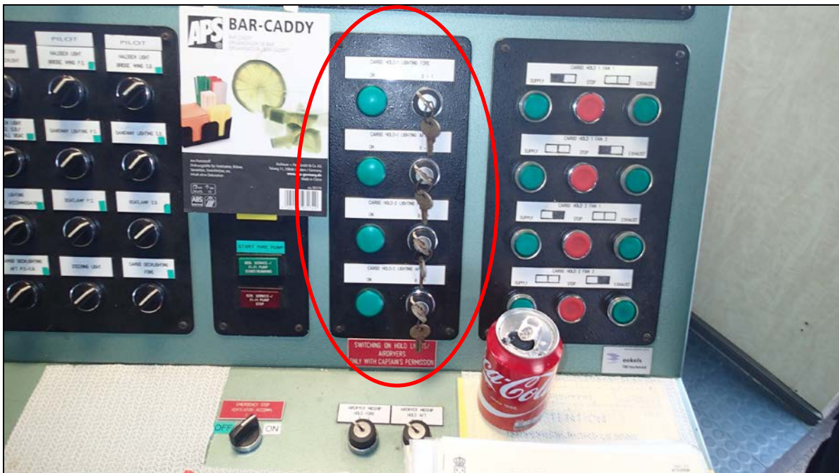
Figure 12: Control panel for the cargo hold lights
