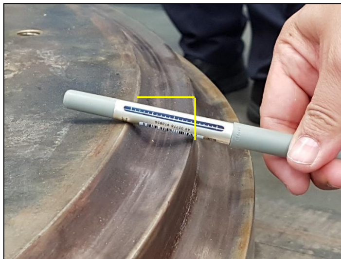
Figure 52: Material removal on cover flange Original condition of the component marked in yellow.
