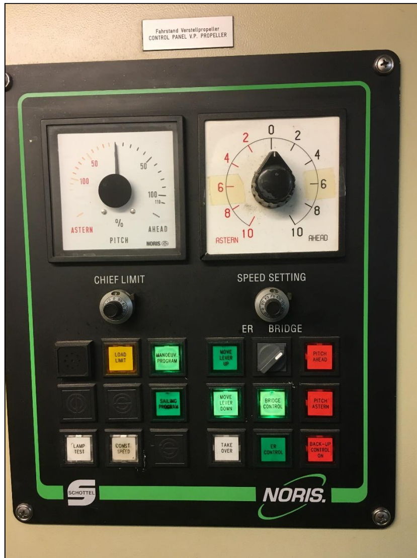
Figure 28: CPP system's control panel in engine room Control was on the bridge when the photograph was taken.
