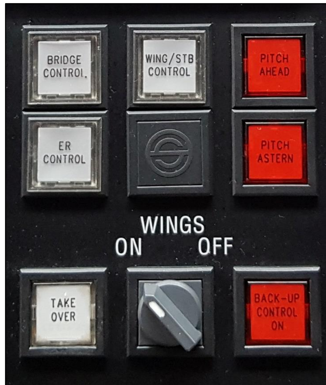
Figure 29: Detail of the CPP system's control panel at the bridge
