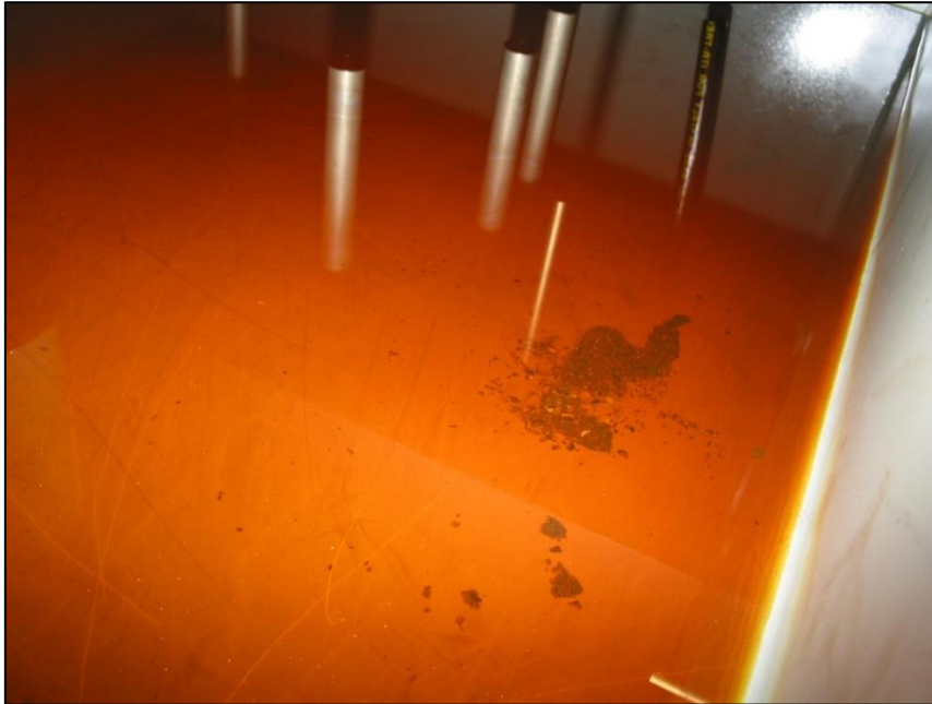
Figure 43: Deposits in the tank of the hydraulic power unit
