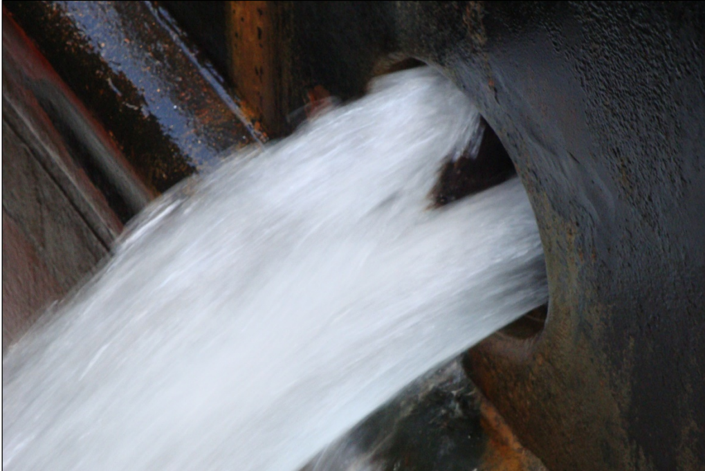
Figure 10: Cooling water discharge outlet (close-up)
