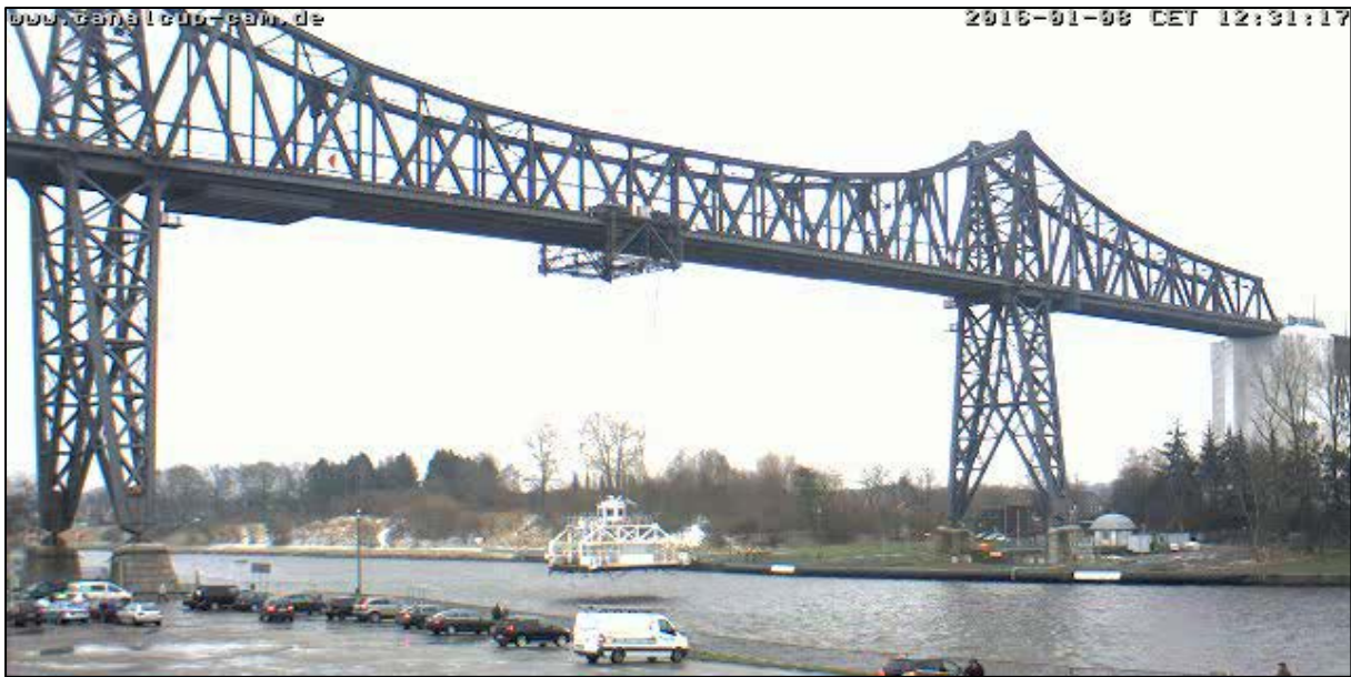
Figure 20: Position of the transporter bridge in daylight after the accident
