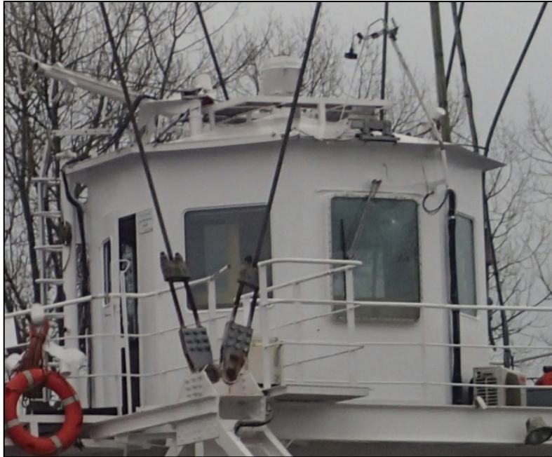
Figure 35: Door on the eastern side and windscreen wiper on the northern side
