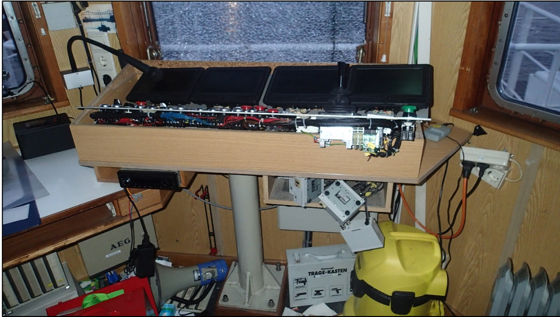
Figure 45: View of the control panel on the northern side
