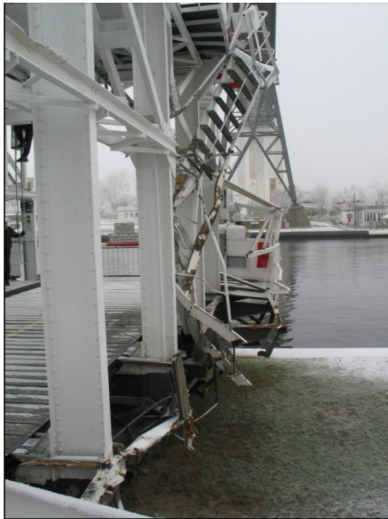
Figure 41: View of the destroyed passenger platform and steps to the control position
