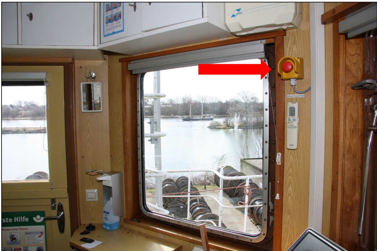
Figure 46: Position of the emergency stop button to the left above the southern control panel
