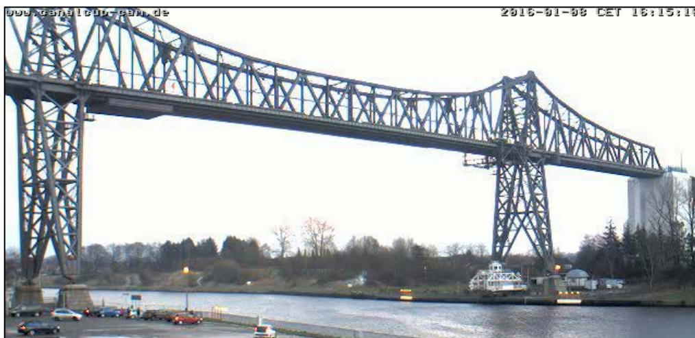
Figure 21: Recovery of the damaged transporter bridge (08/01/2016, 1615)
