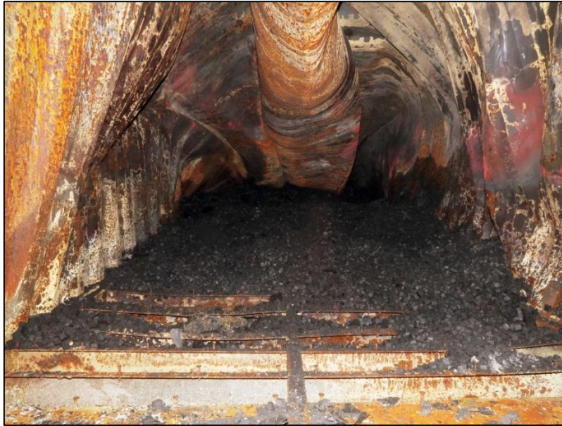
Figure 32: View into the container at slot 120782
