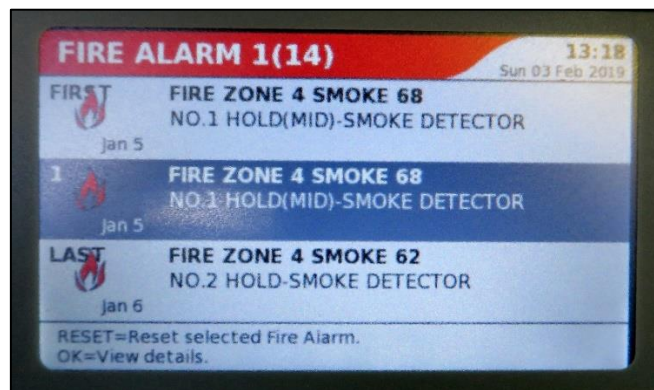
Figure 24: Fire alarm system display
