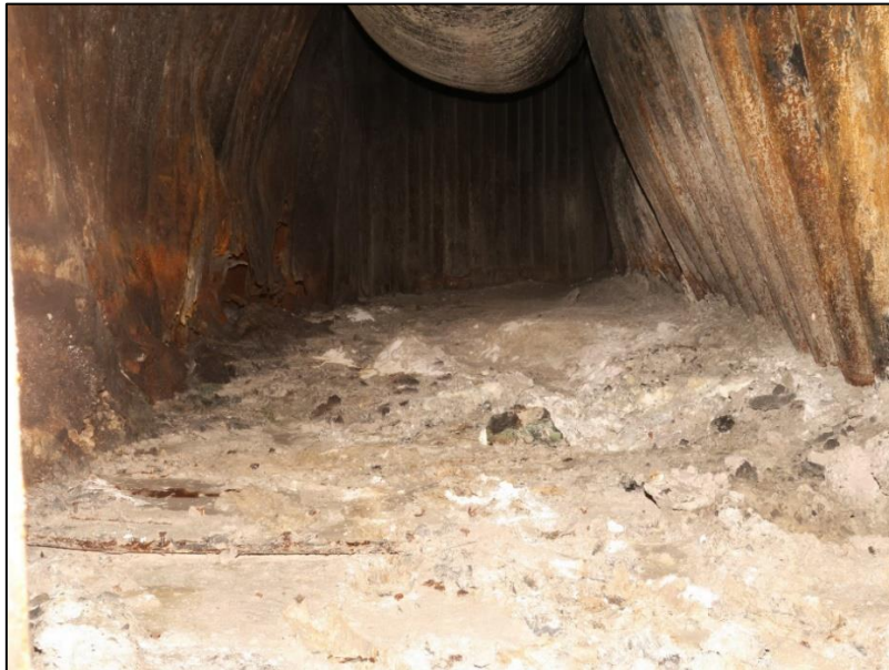
Figure 30: View into the container at slot 120582 Small amount of fire debris; floor completely burnt.
