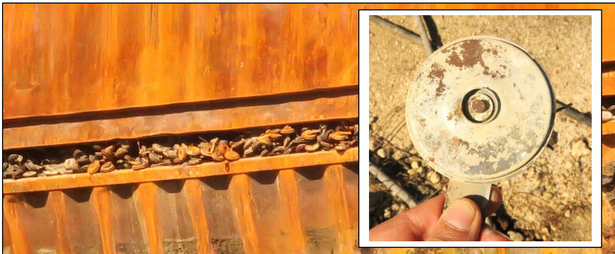
Figure 59: Horn from container at slot 120384
