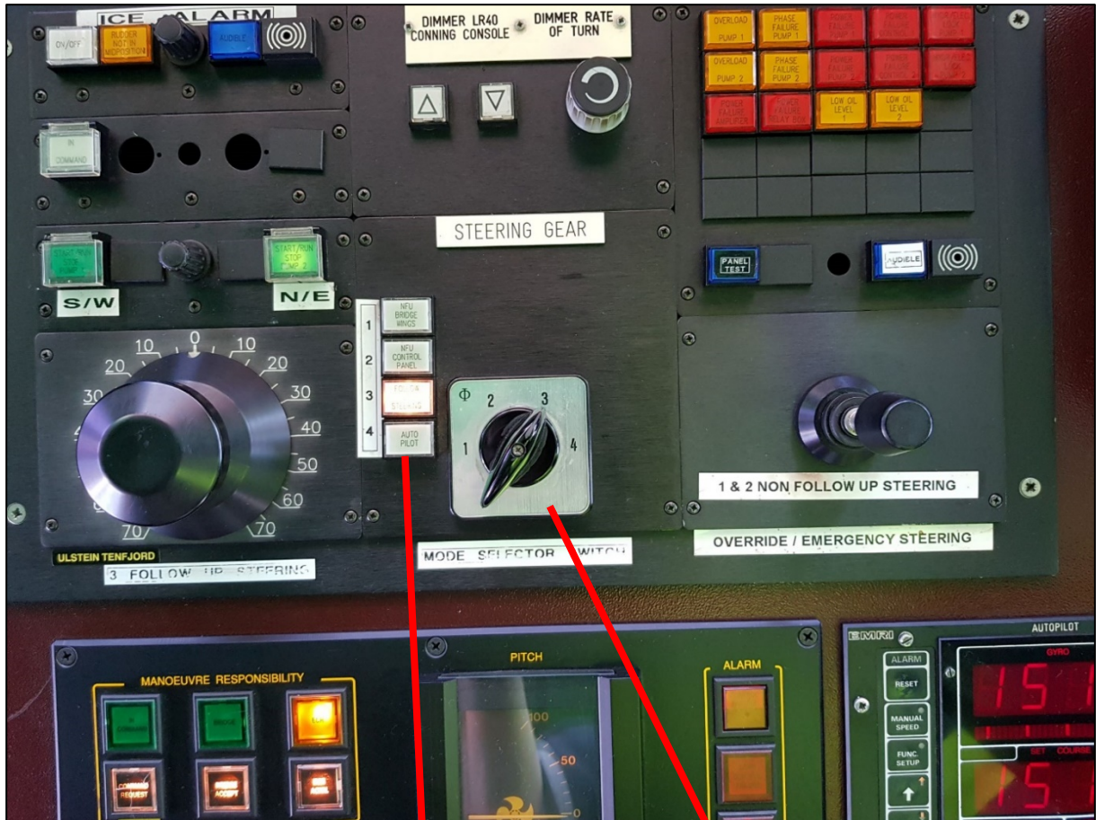
Figure 3: Steering gear control panel
