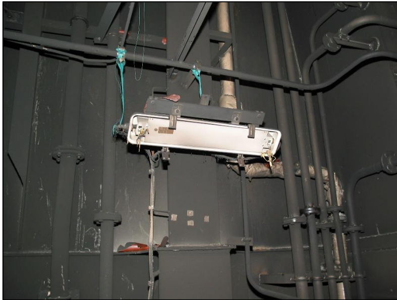
Figure 10: Damage to lights and cables
