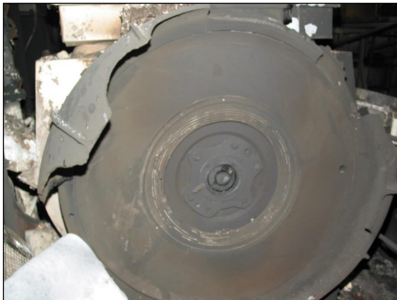
Figure 17: Bearing shield on compressor side
