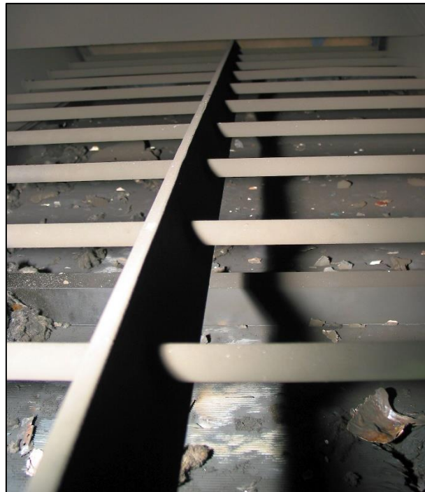
Figure 20: Compressor side of the charging air cooler
