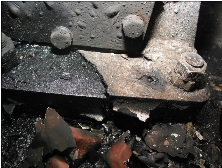
Figure 19: Fractured base of the turbocharger
