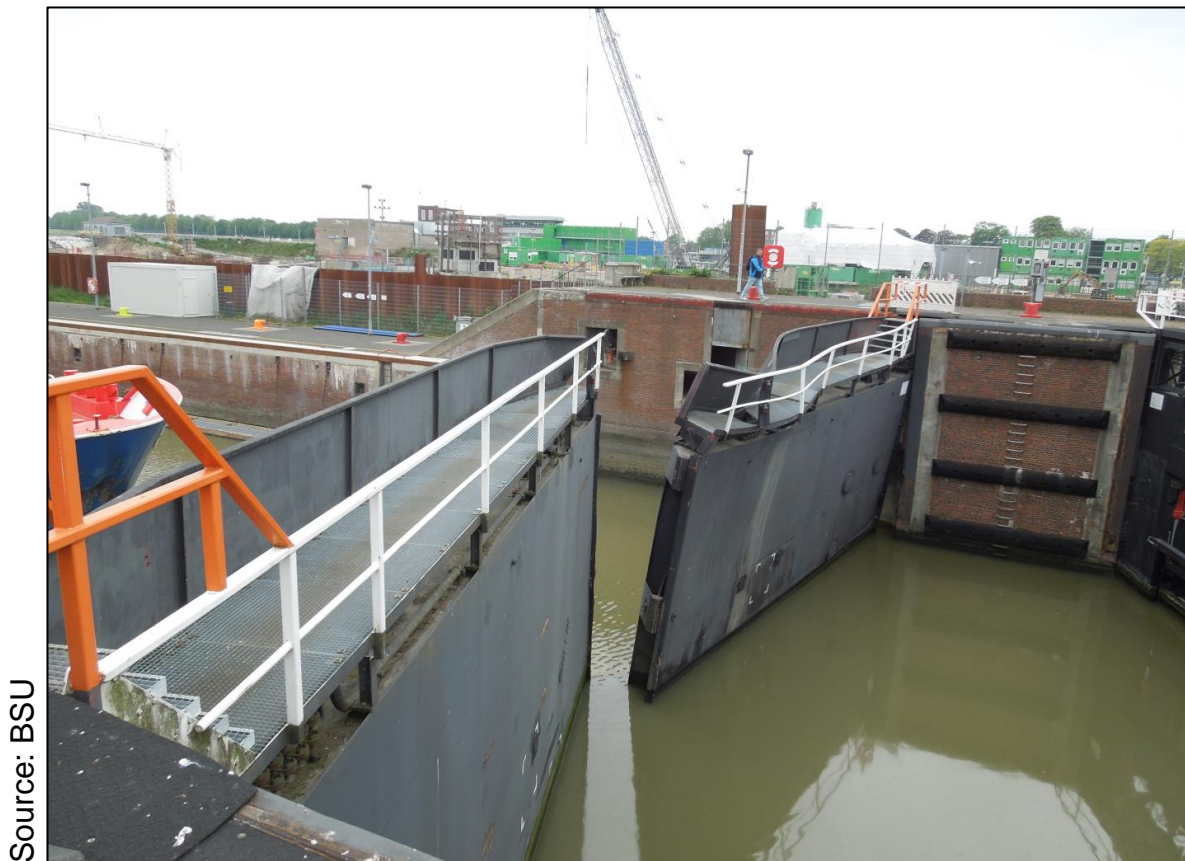
Figure 3: Dented lock gate
