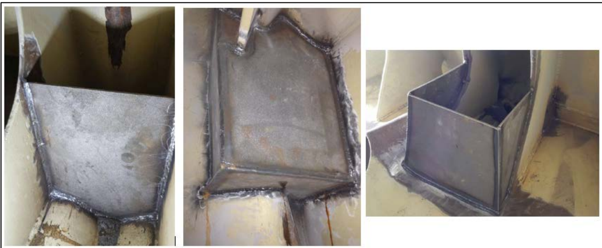
Figure 9: Box structures in the area of the cracks
