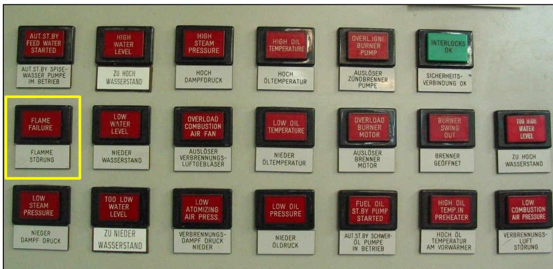
Figure 5: Area A: Alarm panel (extracted from Figure 4) Flame Failure/Flamme Störung indication outlined in yellow.
