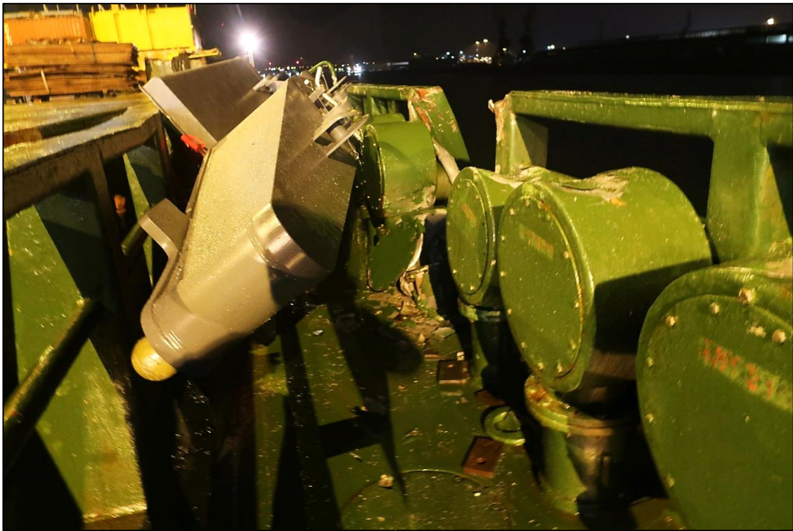
Figure 12: Damage to port-side deck passageway caused by crane 1 (e.g. broken off supporting pad)
