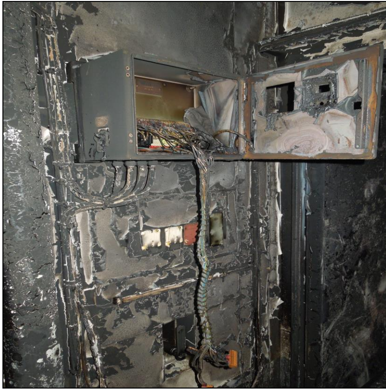
Figure 12: Control valve's switch box with wiring harness hanging out
