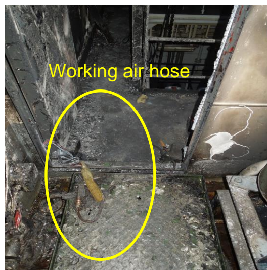
Figure 18: View from the separator room into the engine room An air hose that had been used for clearing the dismantled pipe section can be seen lying on the floor.
