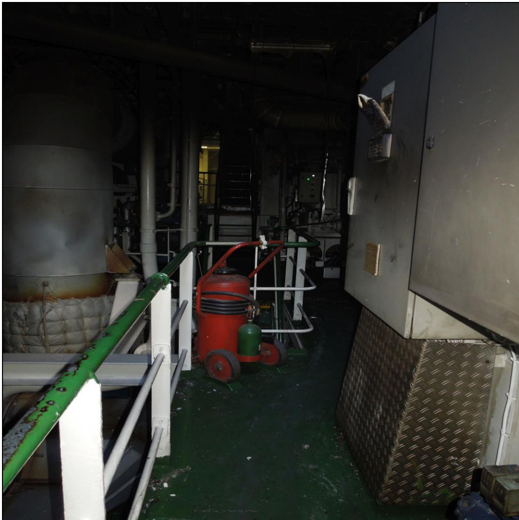
Figure 10: View from the separator room toward the exit of the engine room
