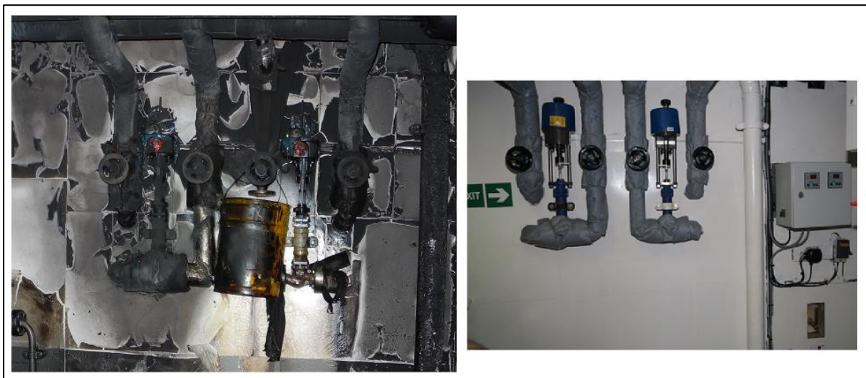
Figure 30: Control valves after the accident on the left and after the repair on the right
