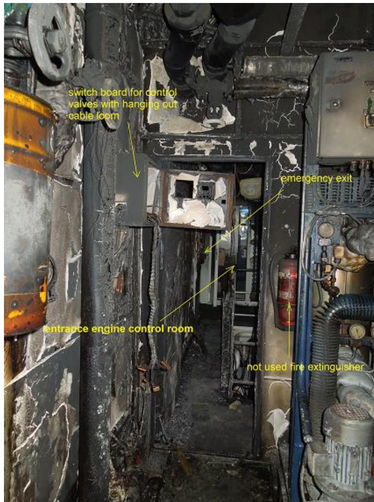
Figure 17: View from the separator room into the engine room The entrance to the engine control room can be seen opposite.
