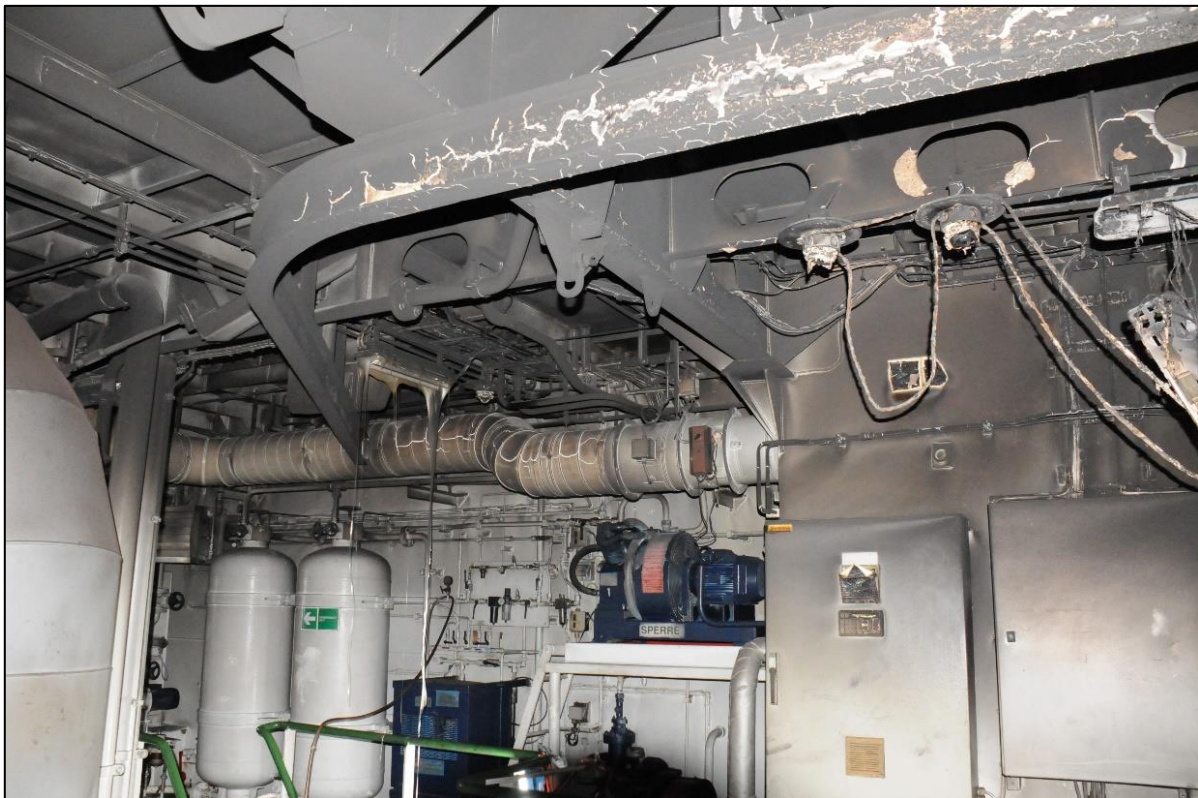
Figure 14: Fire zone beneath the ceiling
