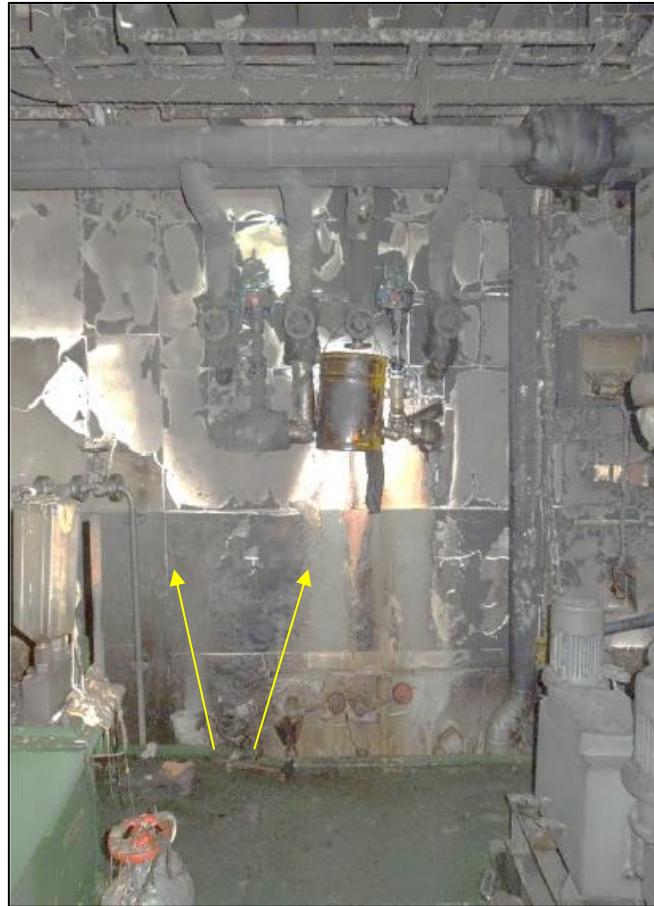
Figure 19: Partial overview of the scene of the fire with opened pipe system
