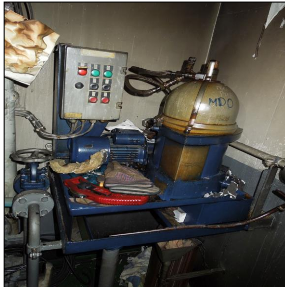
Figure 21: MDO separator (less than 2 m away from the position at which the fire broke out)
