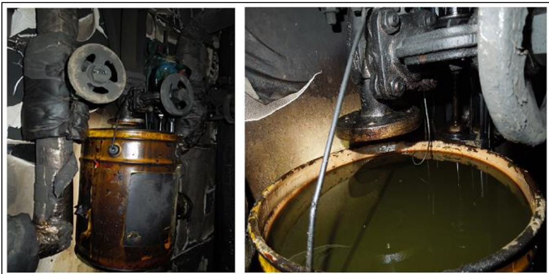
Figure 16: Bucket filled with thermal oil below the valve
