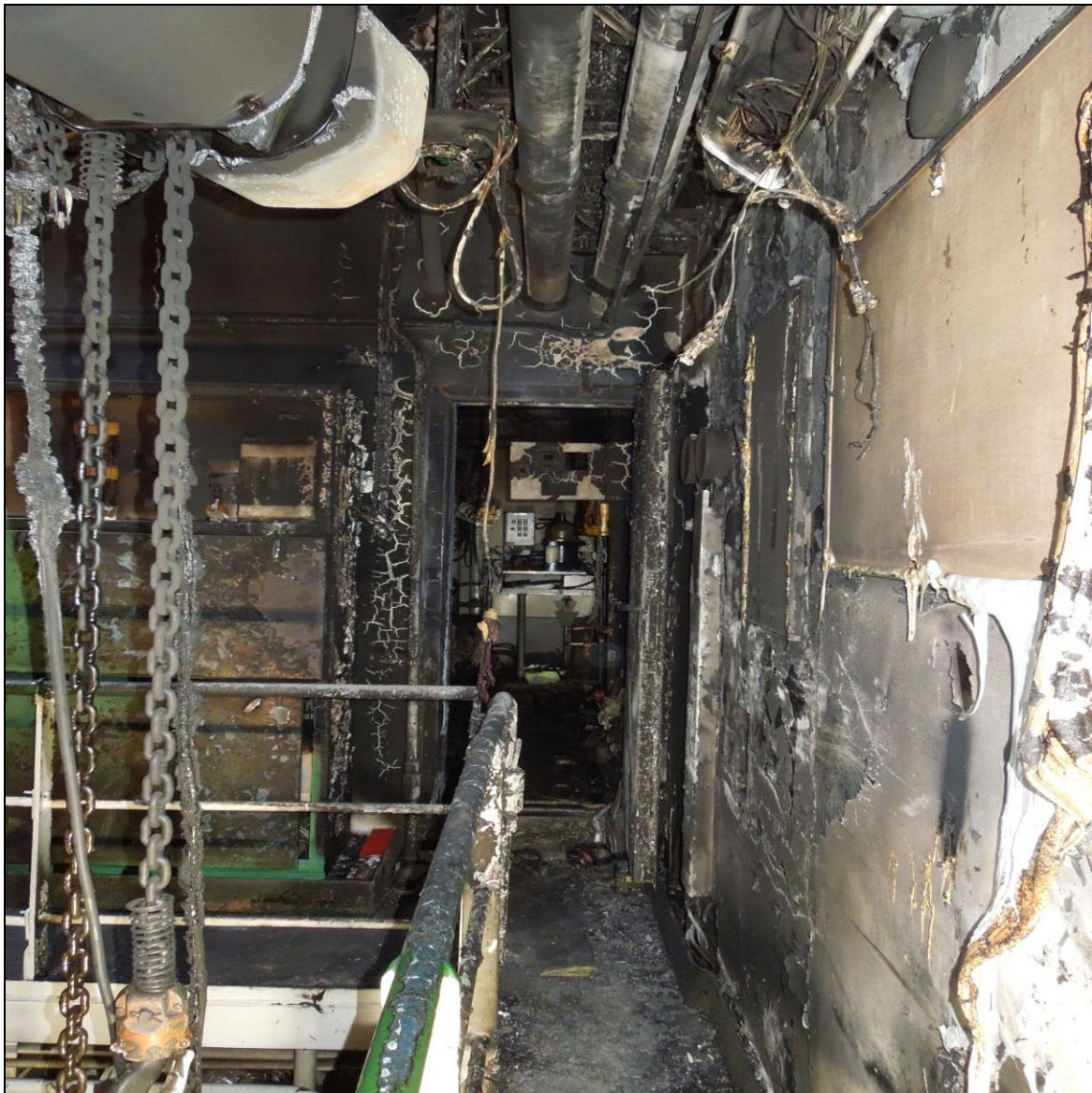
Figure 11: View from the engine control room opposite into the separator room
