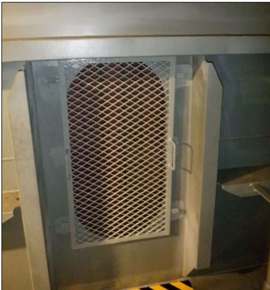
Figure 26: Secured Access to Cargo Hold with a Risk of Falling 78
