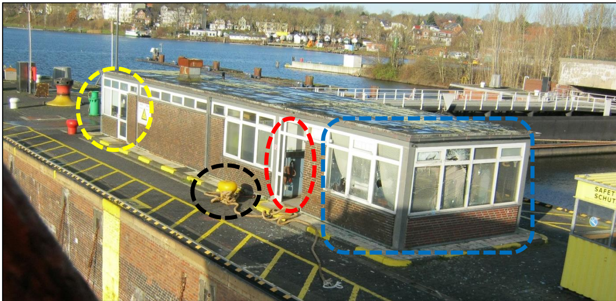
Figure 3: Service building on the lock wall with damaged windows 5
