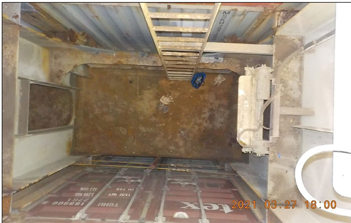
Figure 5: View of the 4th Stringer Deck in Cargo Hold No. 3 from Above; Scene of the Accident 15
