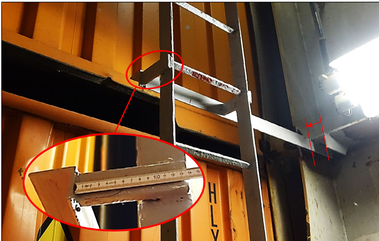
Figure 18: Moved Ladder Support Strut in CH3 111
