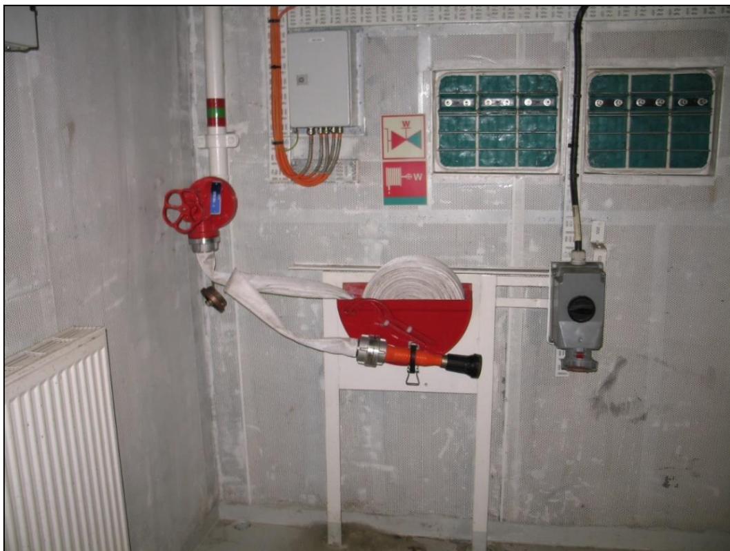
Figure 35: Equipment prior to fire
