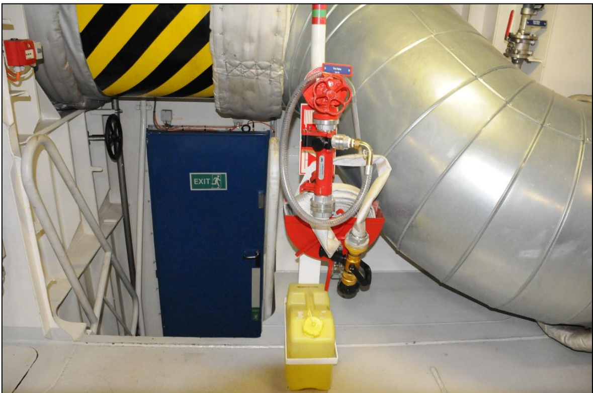
Figure 46: Hydrant station with foam/wetting agent
