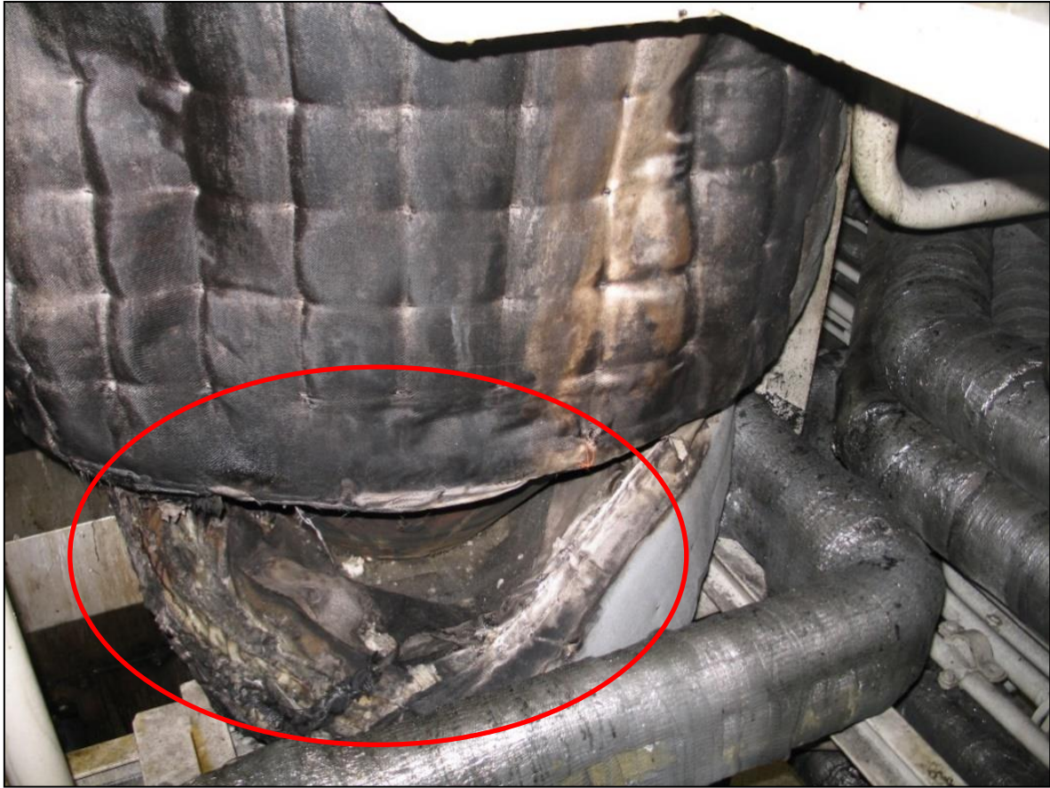
Figure 18: Burn marks on insulation mats of exhaust pipe
