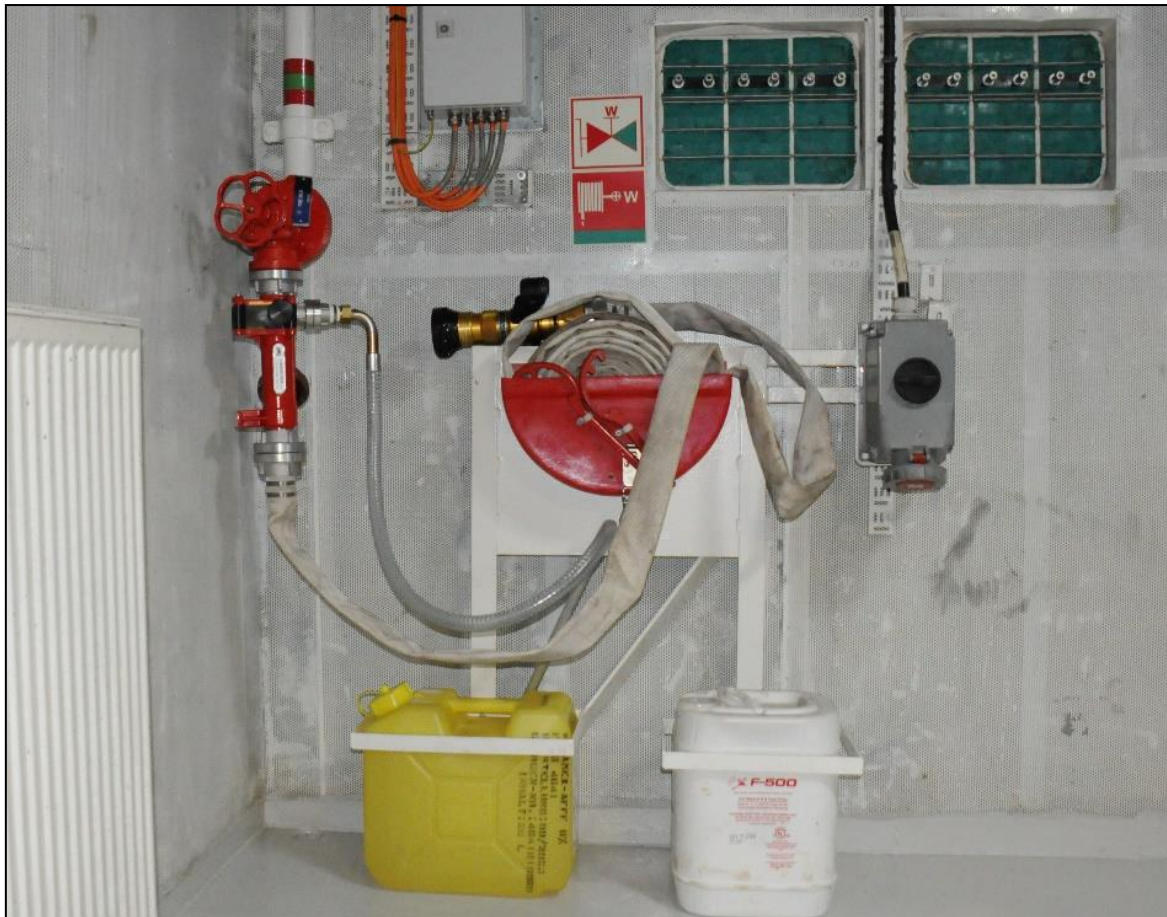
Figure 36: Equipment after fire
