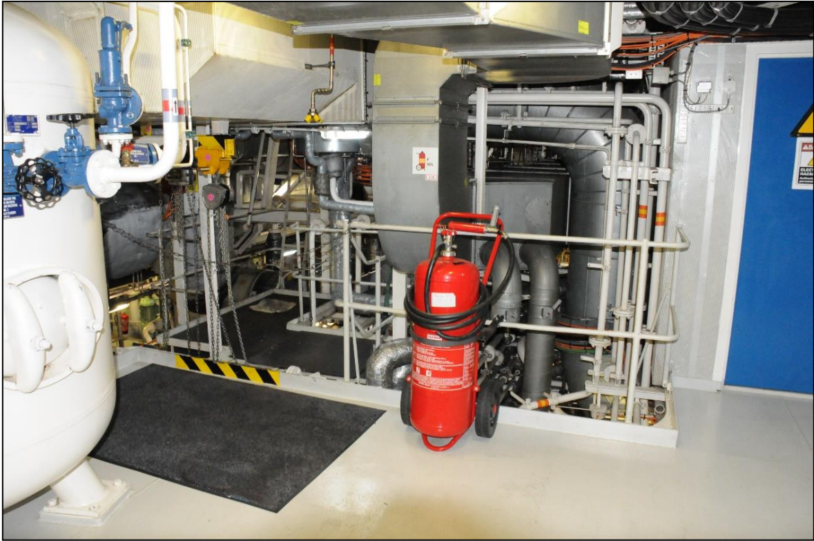
Figure 32: Foam trolley (in risk area)
