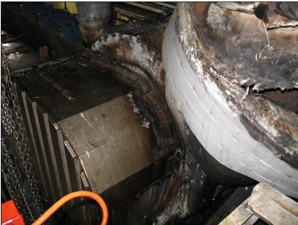
Figure 22: Fire damage to exhaust side insulation in area of turbocharger
