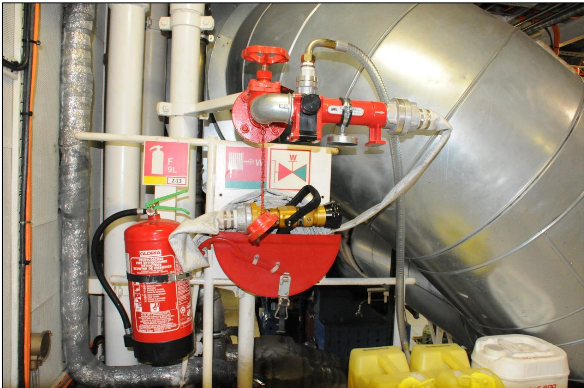
Figure 44: Hydrant station (risk area) with permanently installed admixture/inductor and turbo jet pipe
