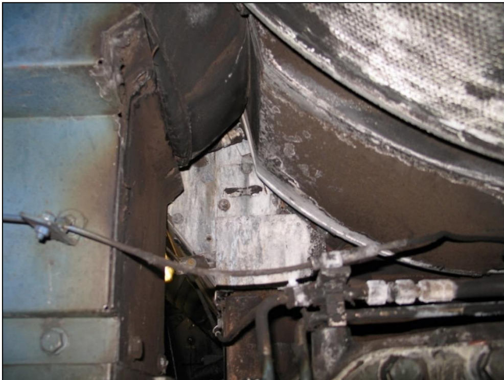
Figure 20: Fire damage to turbocharger insulation (air side)
