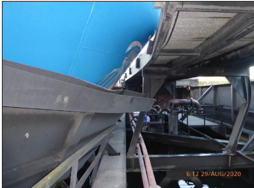
Figure 7: Damage to the lock gate (close-up 1) 23
