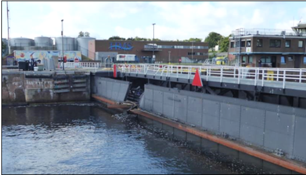
Figure 9: Damage to the lock gate (general view) 24
