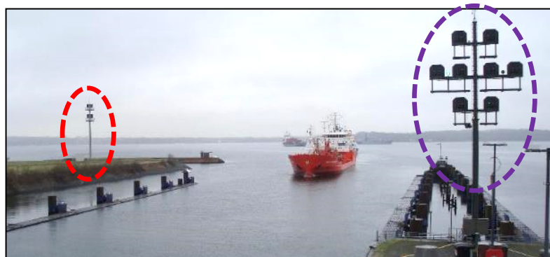
Figure 39: Signal installations (entries into the approach channel and the Neue Schleuse)
