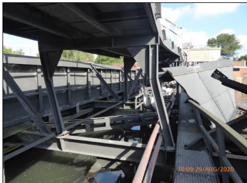
Figure 8: Damage to the lock gate (close-up 2)
