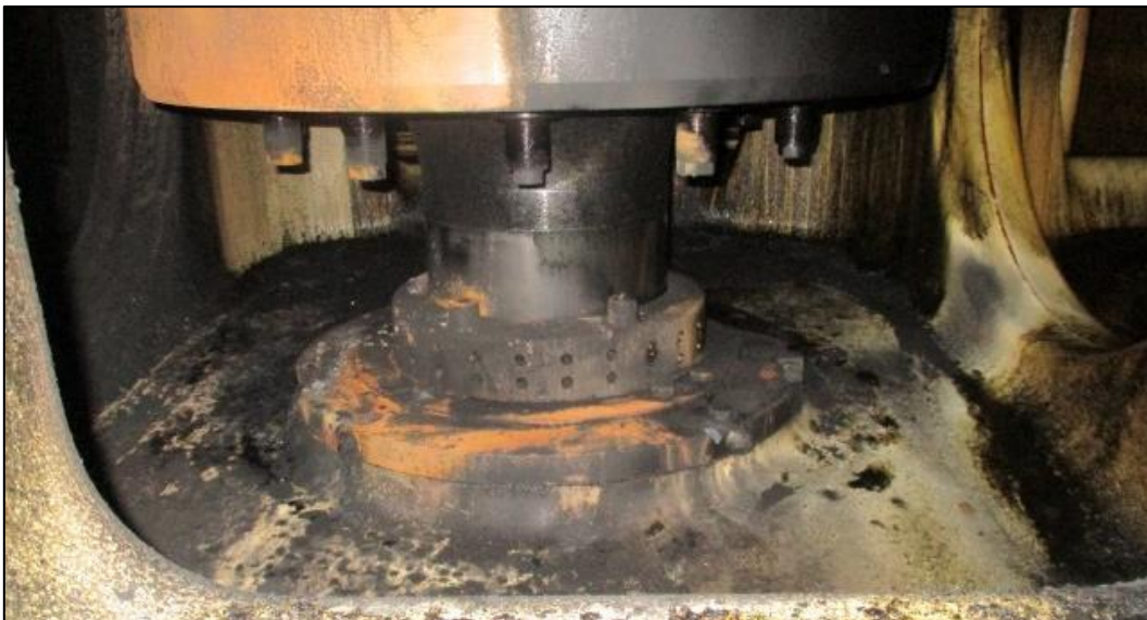
Figure 4: Stuffing box area of an affected cylinder 16 with traces of rust from the extinguishing water
