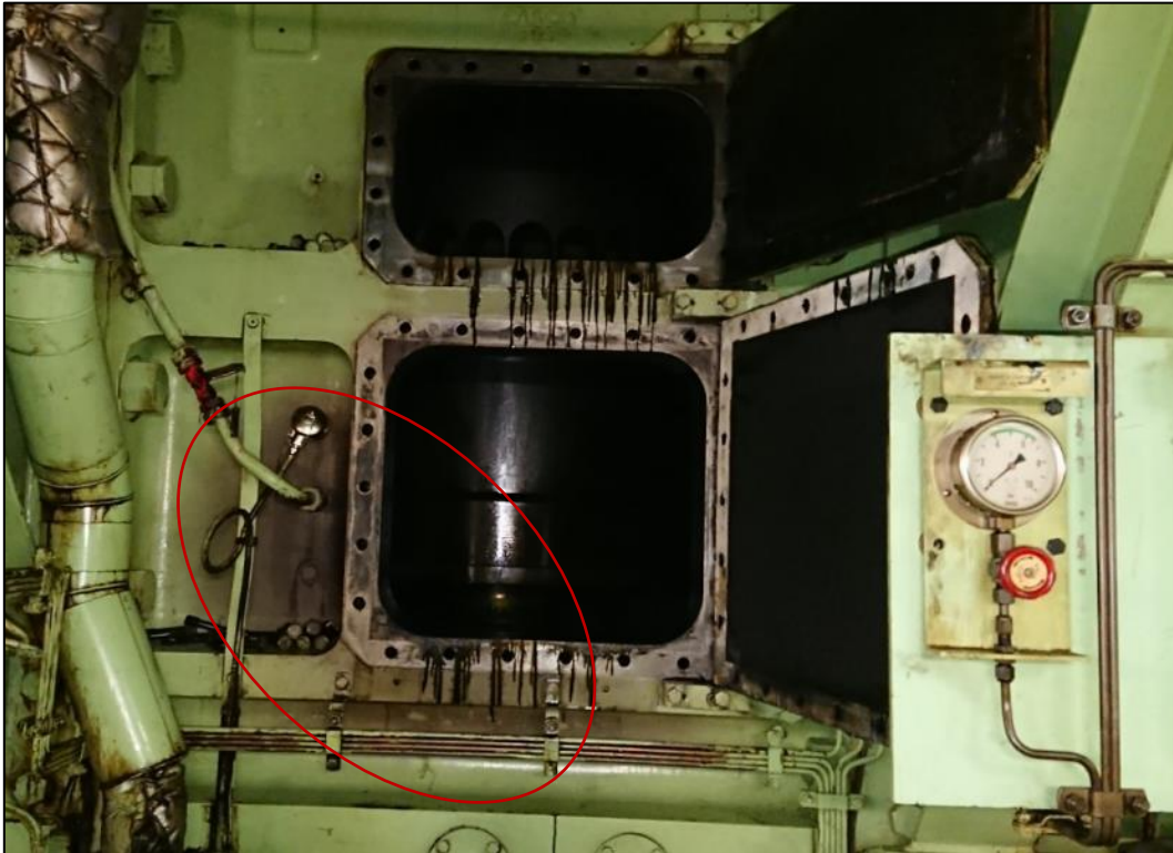
Figure 5: Paint on the main engine discoloured by high temperatures next to the scavenge air duct inspection hatch of a cylinder affected by the fire
