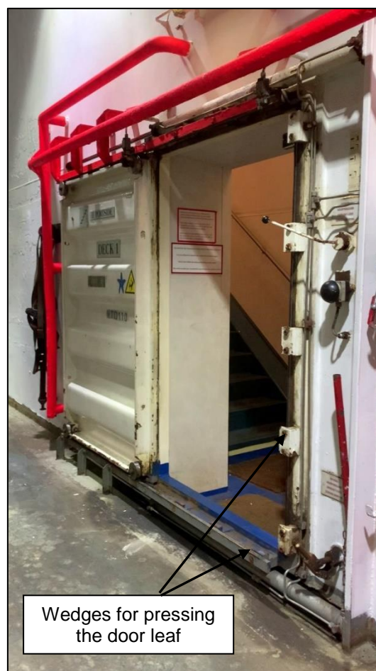
Figure 5: Watertight door number 110 on deck 1 in the open condition 8
