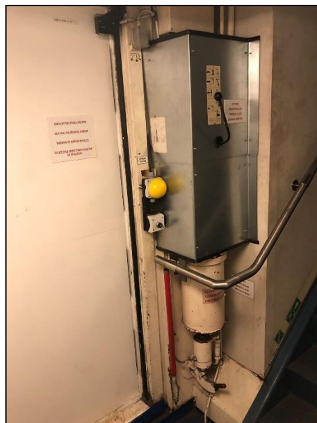
Figure 17: Watertight door number 108 with the new extended handrail reaching around the corner 22
