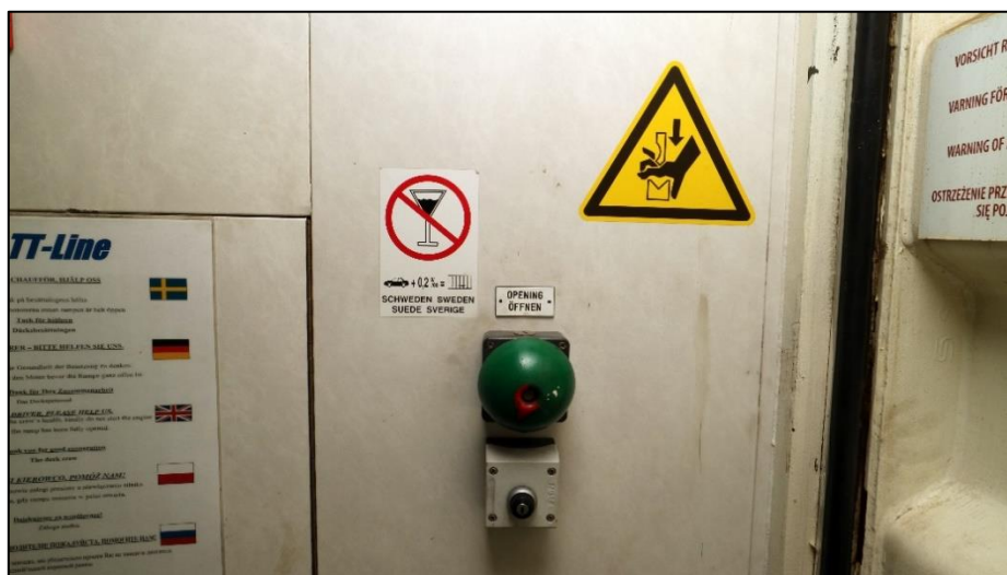
Figure 9: Pushbutton for opening the door and 'Risk of Crushing' warning sign 12
