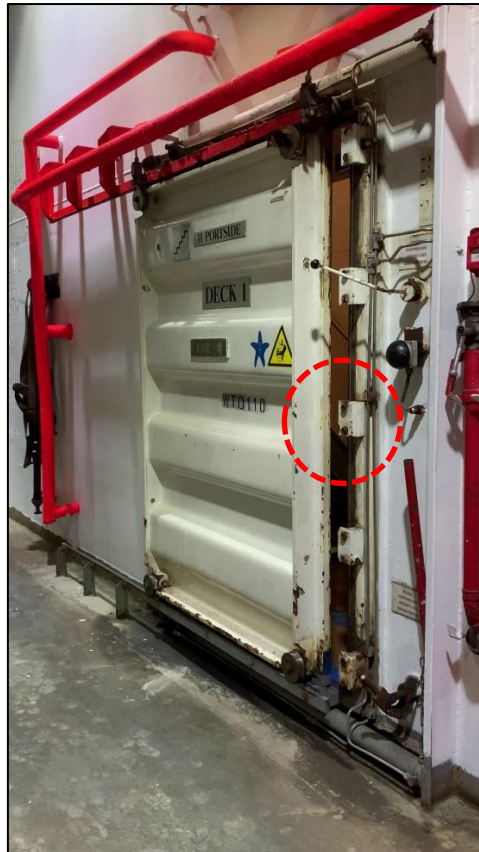
Figure 13: Assumed location at which the injury occurred 16
