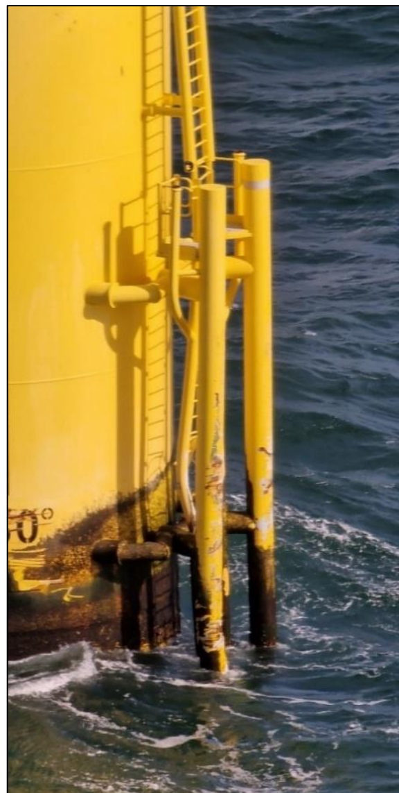
Figure 2: Struck wind turbine in detail 5
