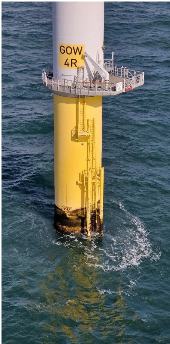
Figure 1: Struck wind turbine in overview
