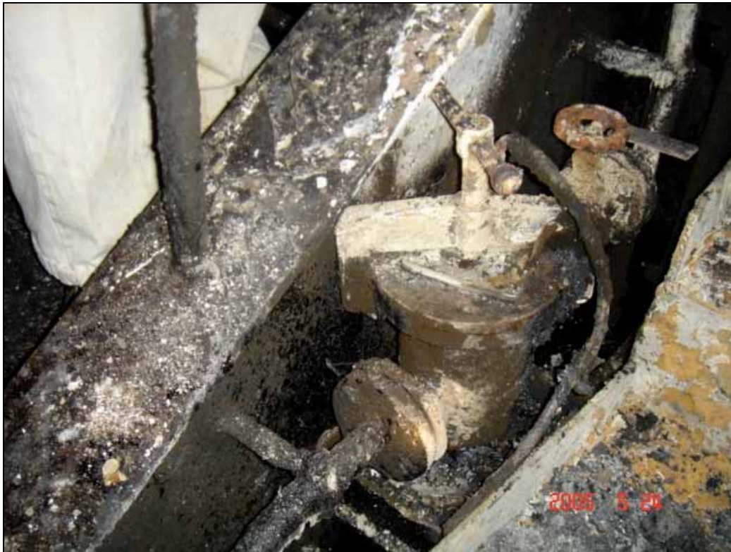
Figure 7: Diesel oil filter in the emergency system
